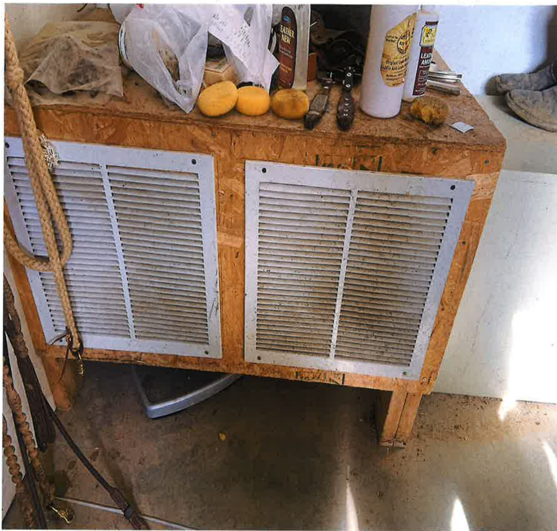
Fig. 5 – Second heater in closet area of shed used for heating.
