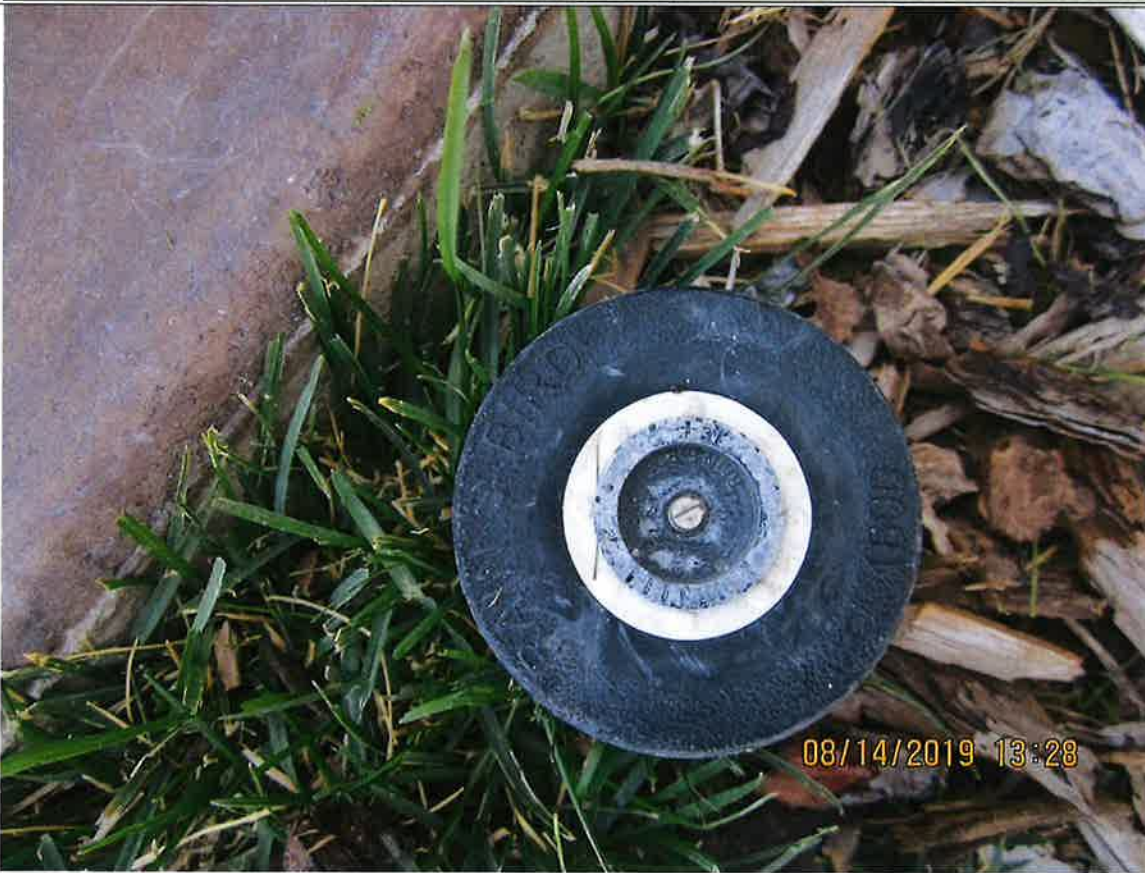
Figure 6. Rainbird 1800 pop up sprinklers used to water the lawn area.
