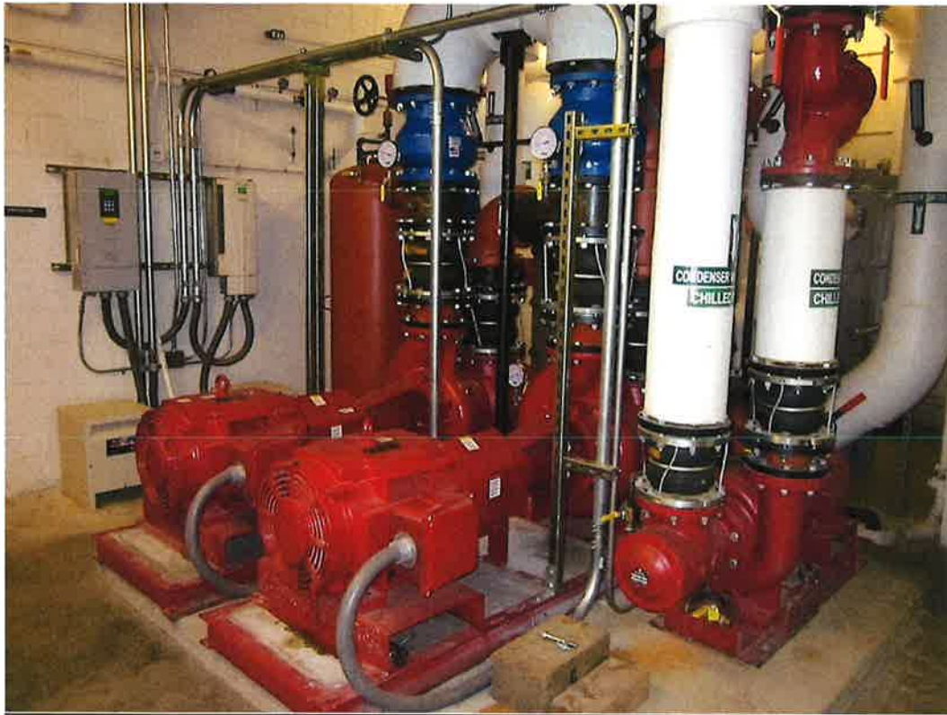
Figure 1: Part of Heating and cooling distribution system where heat exchangers are located
