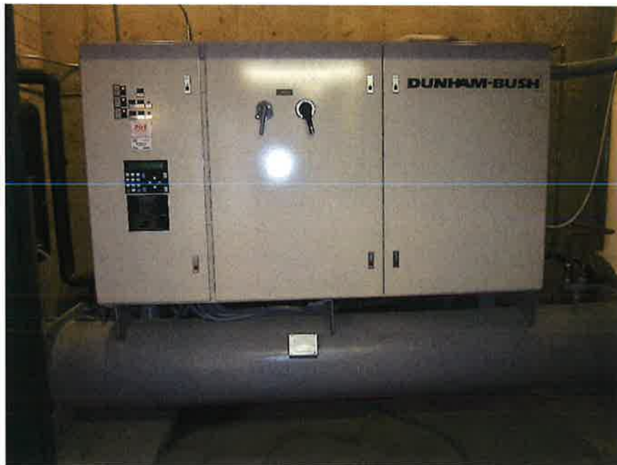
Figure 4: Chiller for entire system housed in separate room adjacent to distribution network
