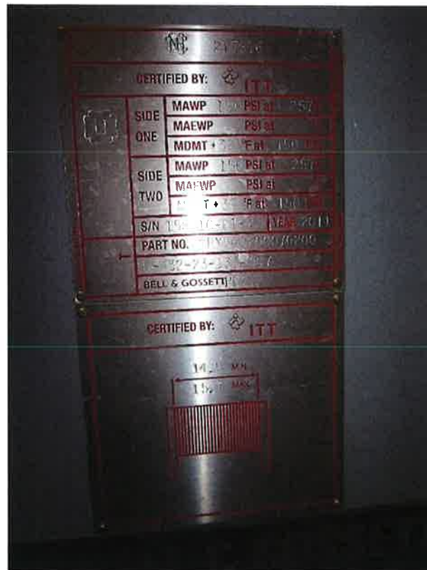
Figure 5: Tag on heat exchanger
