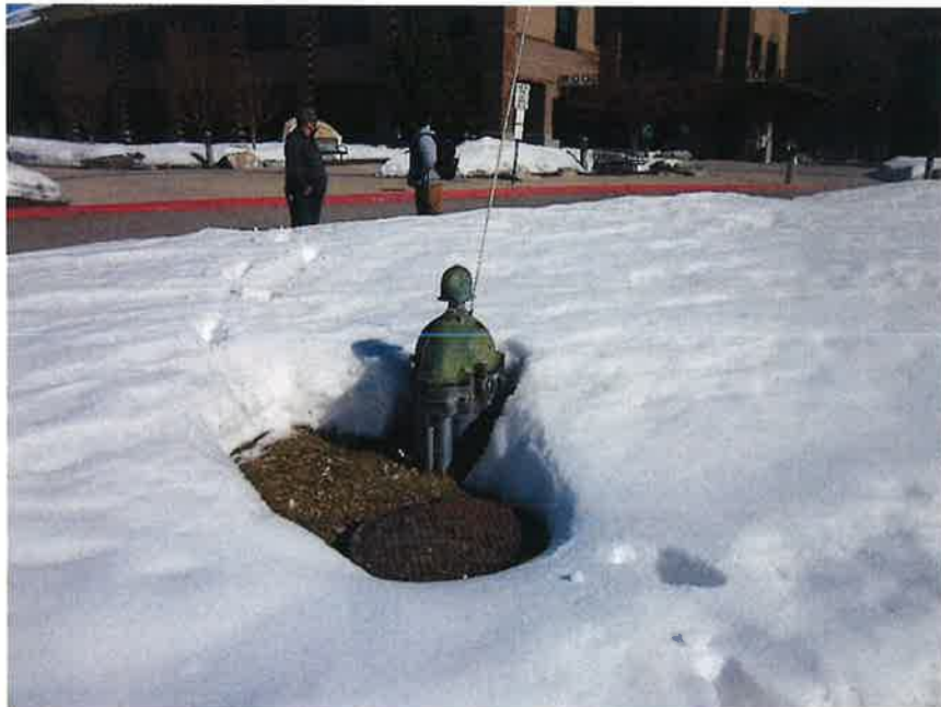
Figure 8: Production well #2, high school and maintenance staff
