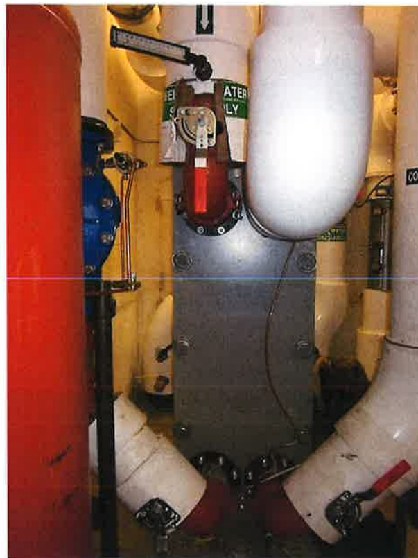
Figure 2: One of Two heat exchangers
