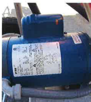
Portable 3 Hp pump used for cleaning outdoor tanks and equipment.
