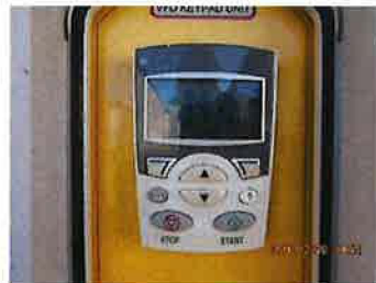
Digital keypad unit at power panel. 65.7 PSI observed at site visit.
