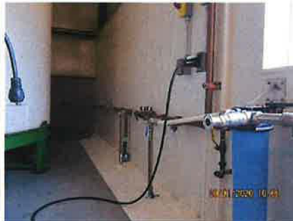
1" outlet nozzle used for cleaning bottling building and equipment.
