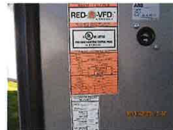
Inside of power panel showing pump info.
