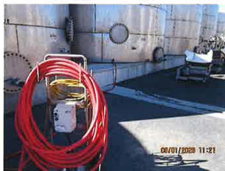
Portable pump connected to red hose, attached to yard hydrant in background. Apple totes seen in background too.
