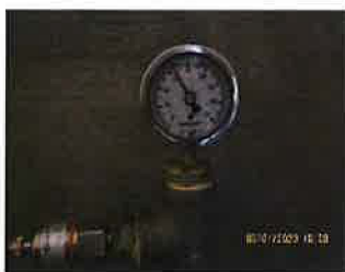
Pressure gage on 1 1/2" pipe inside of bottling building shows approx. 66 PSI.
