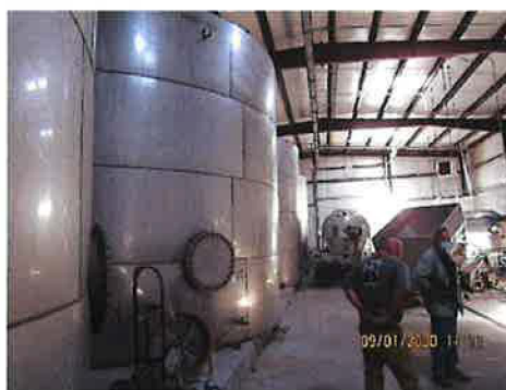
Holding tanks in pressing building. Portable pump to increase pressure for cleaning can be seen in bottom left.
