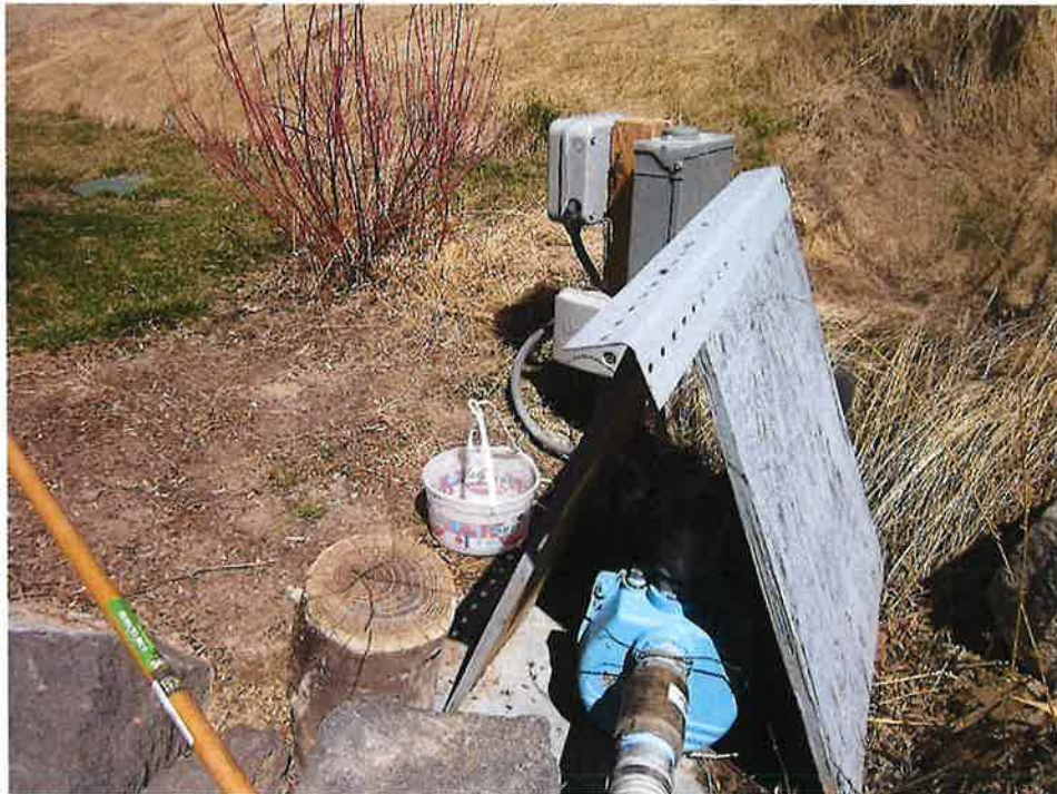
Figure 3: 2Hp pump for irrigation and waterfall
