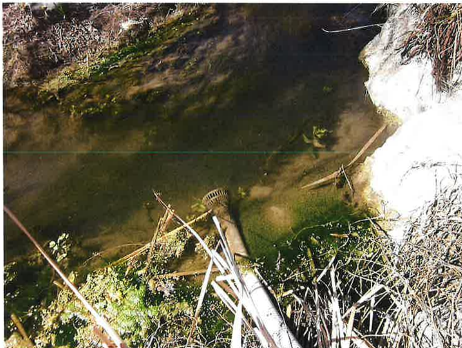
Figure 4: 2" line diverting water from Duck Creek to pump
