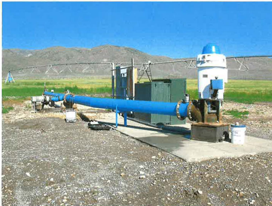
Photo 4. Pump motor and well right center, Polysonic flow meter installed on mainline left center of photo.
