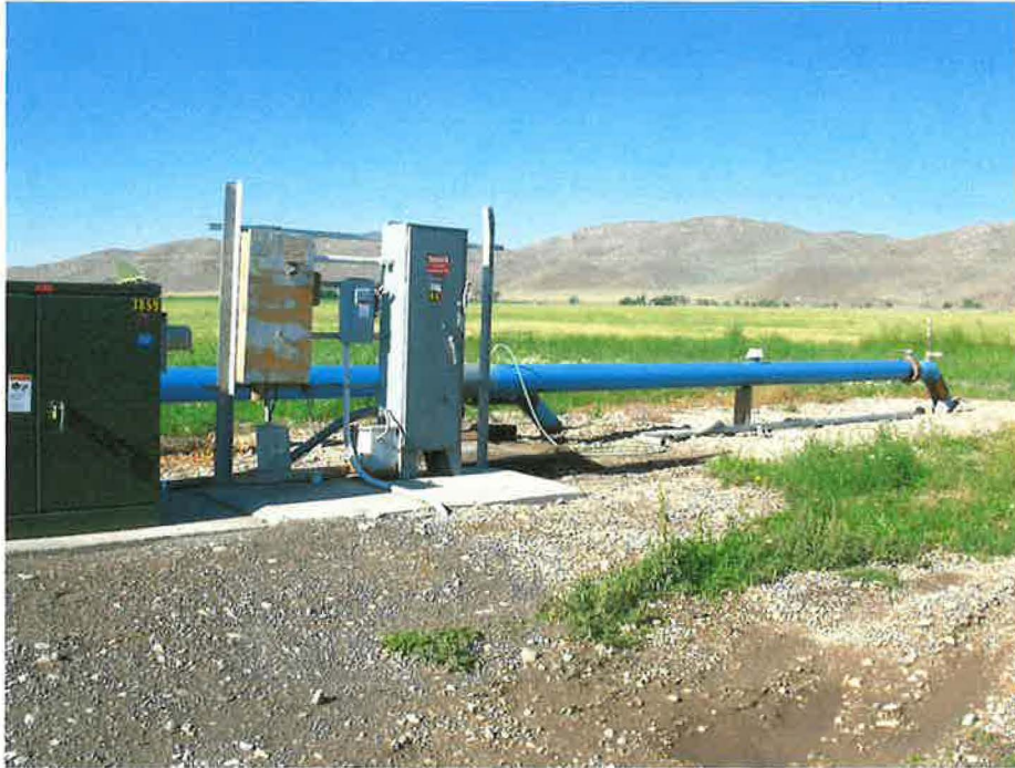
Photo 1. Electrical control panel for well pump on right, booster pump on left. Twelve inch mainline discharges to the right.
