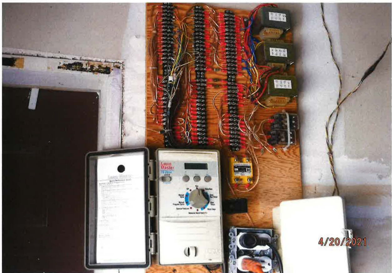
IRRIGATION SYSTEM CONTROL PANEL
