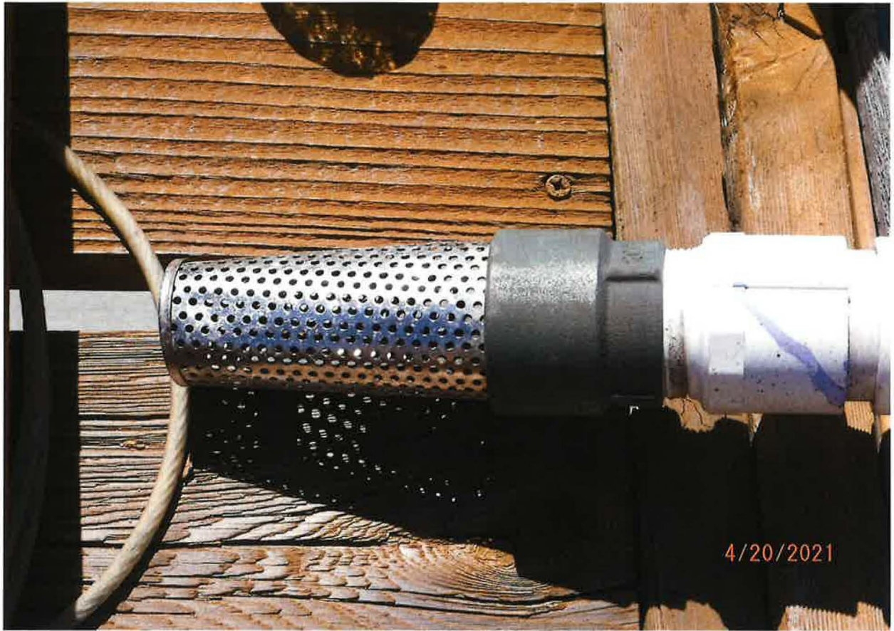
SCREENED INTAKE PIPE AT POD
