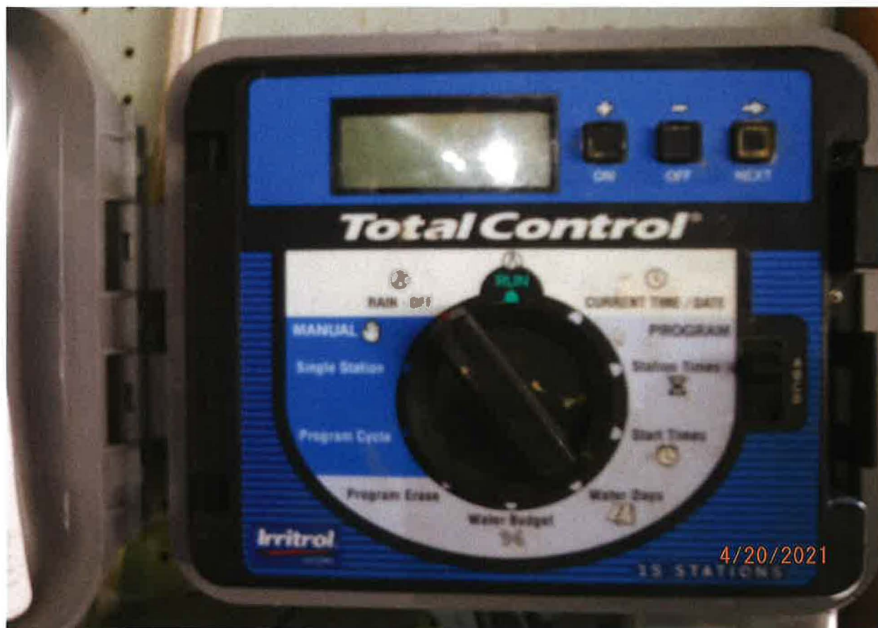
IRRITROL SPRINKLER CONTROL PANEL
