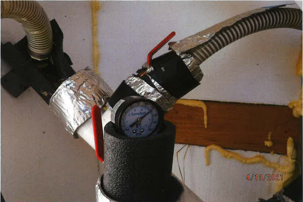
POWER POU – SYSTEM OPERATION STARTS AT 70 PSI, AND DROPS TO 15 PSI BEFORE APPLICANT SHUTS SYSTEM OFF
