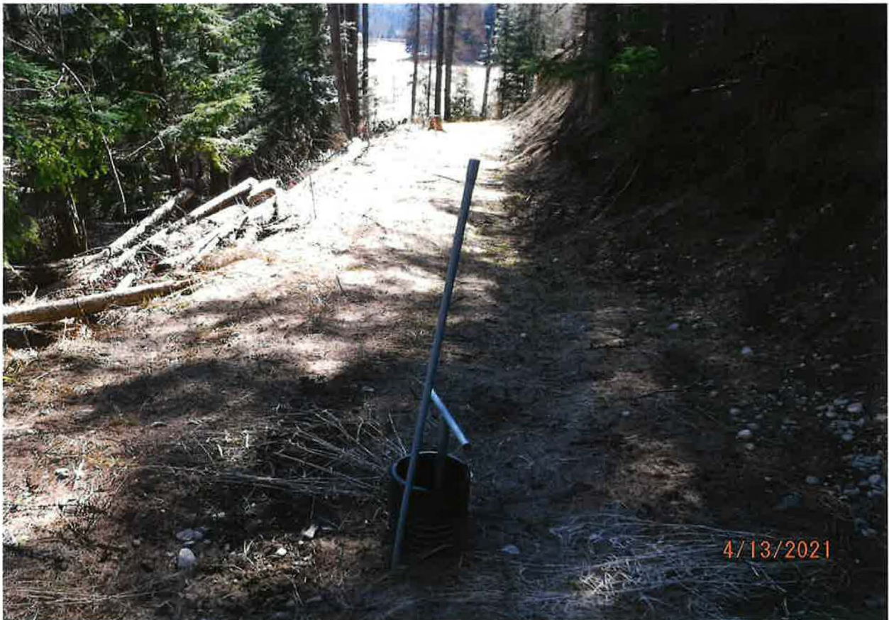
MANUAL VALVE OPERATION FOR HYDRO-POWER 2 INCH POLY PIPE – LOCATED AT POD
