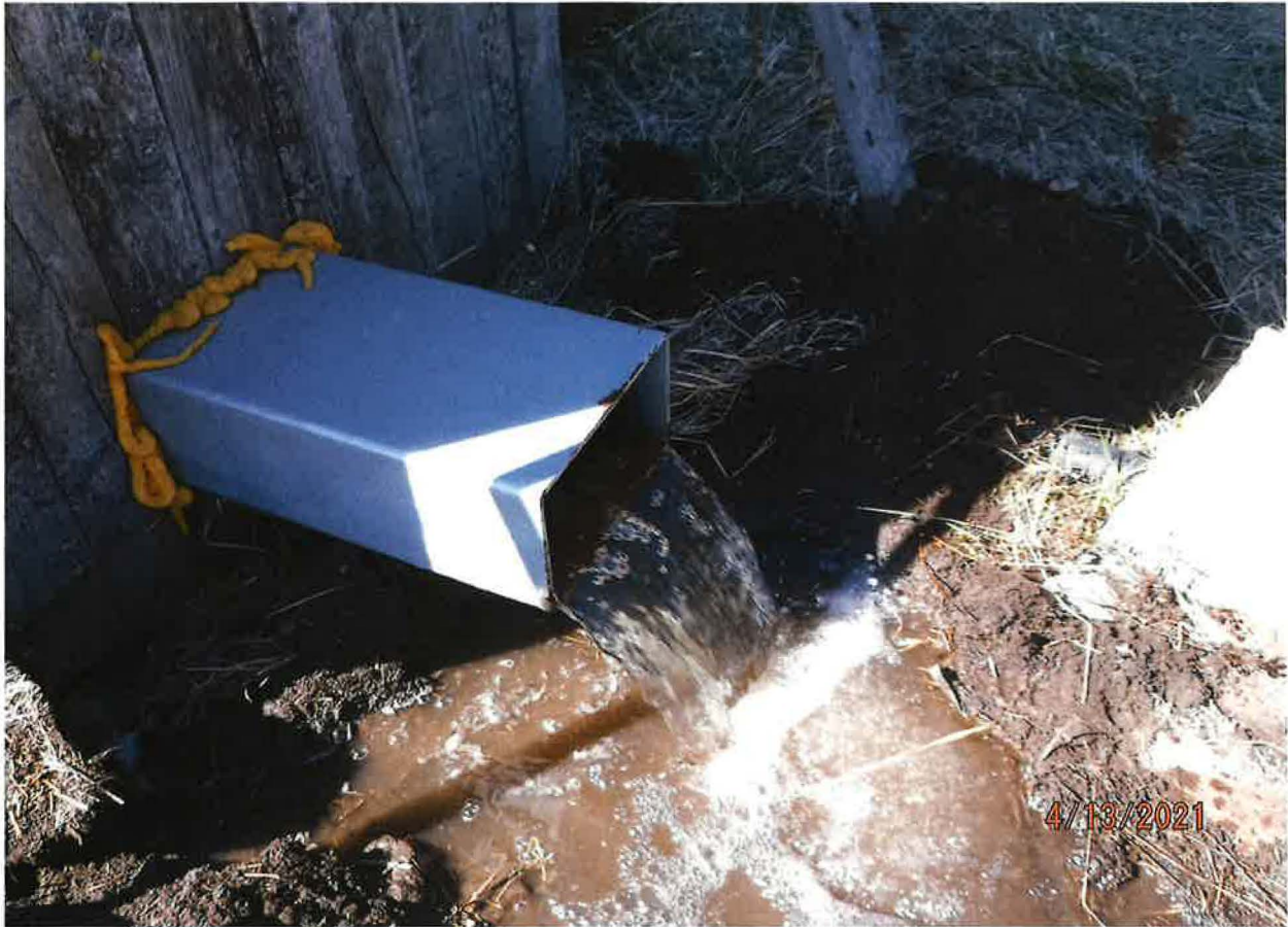
OVERFLOW DISCHARGE FROM HYDRO-POWER UNIT
