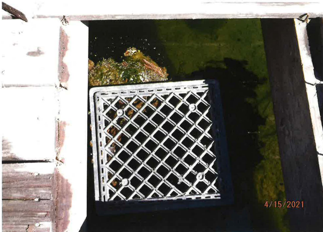
OVERFLOW DISCHARGE PIPE WITH DEBRIS COVER
