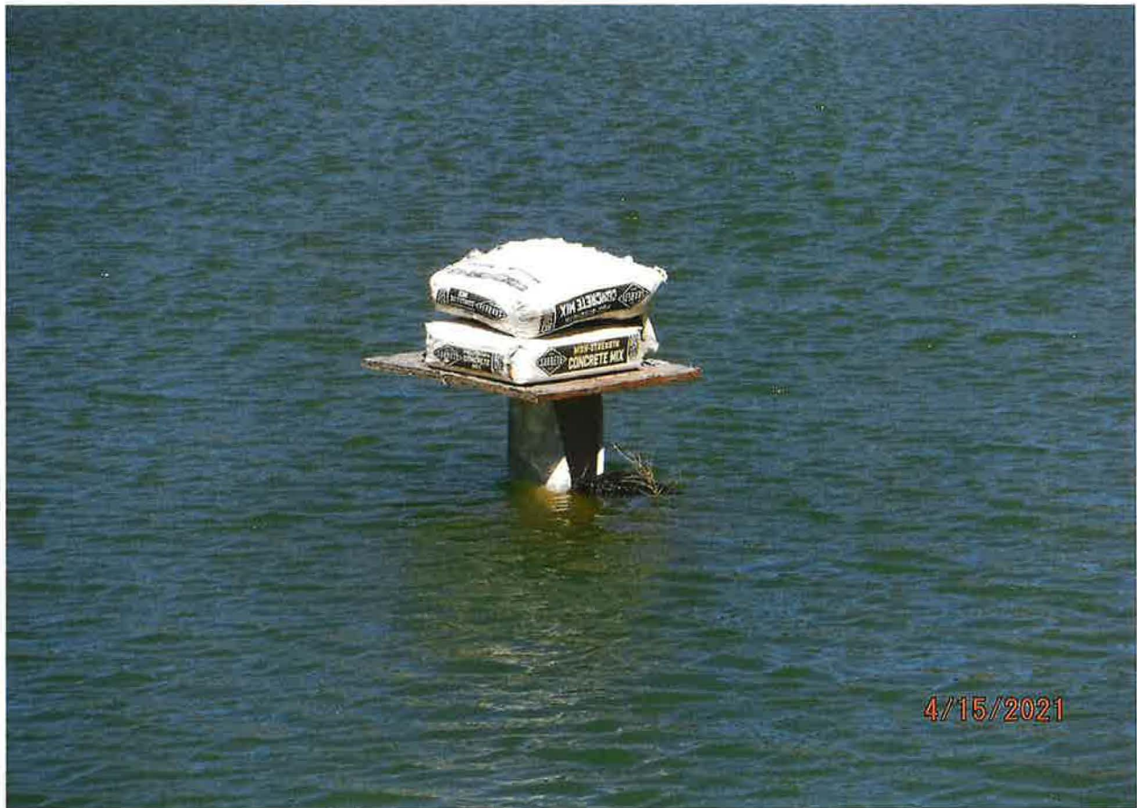
OVERFLOW DISCHARGE PIPE
