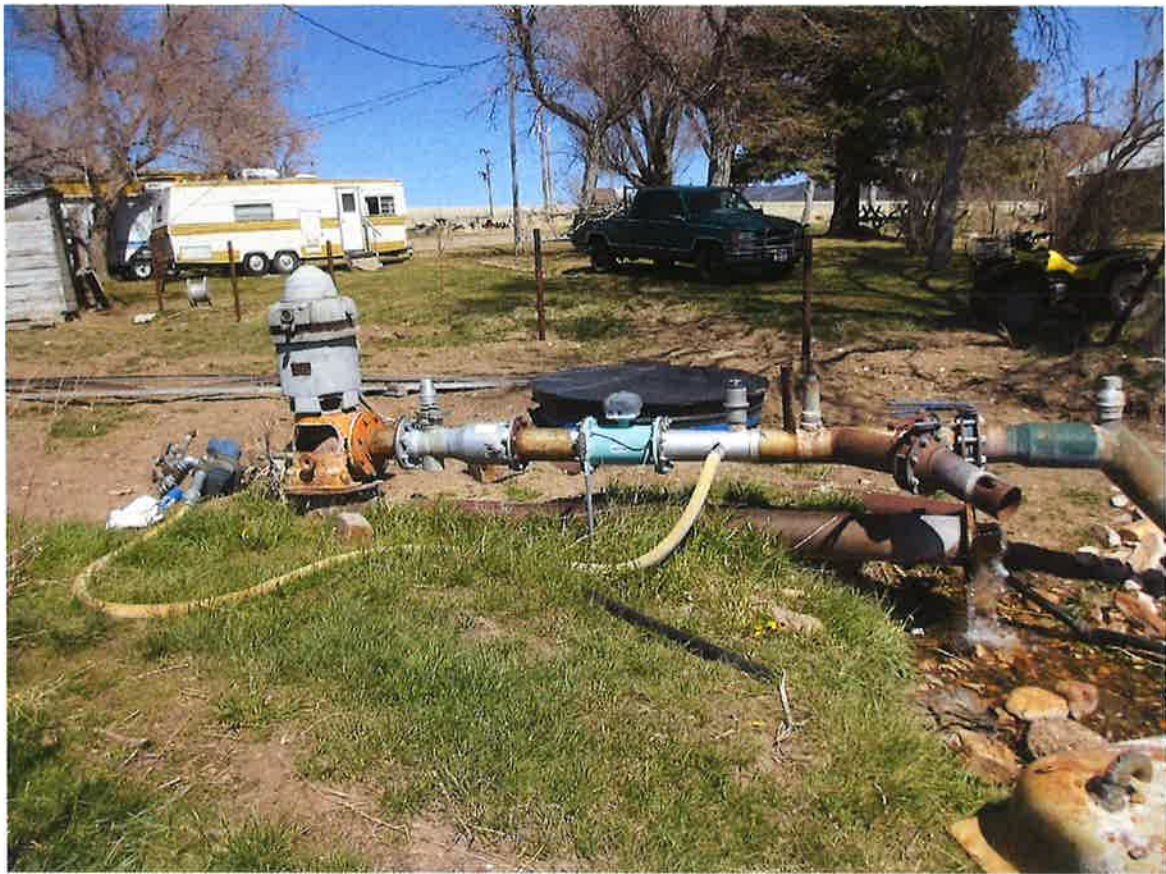
Point of Diversion – Artesian Well
