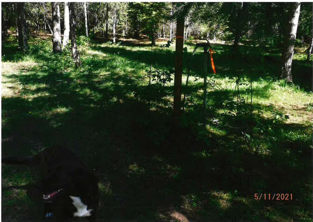
IRRIGATION BY FROST FREE HYDRANTS (7EA) AND HOSE-TO-SPRINKLERS
