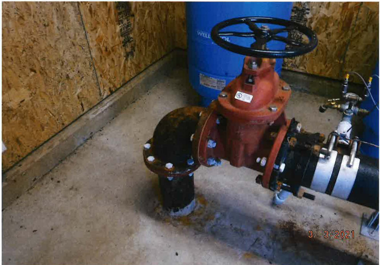
WATER SYSTEM PIPE FROM WELL
