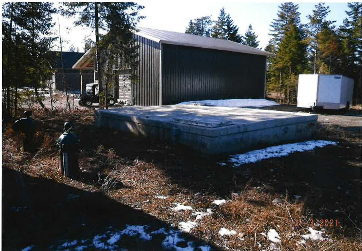
17,000 GALLON STORAGE RESERVOIR
