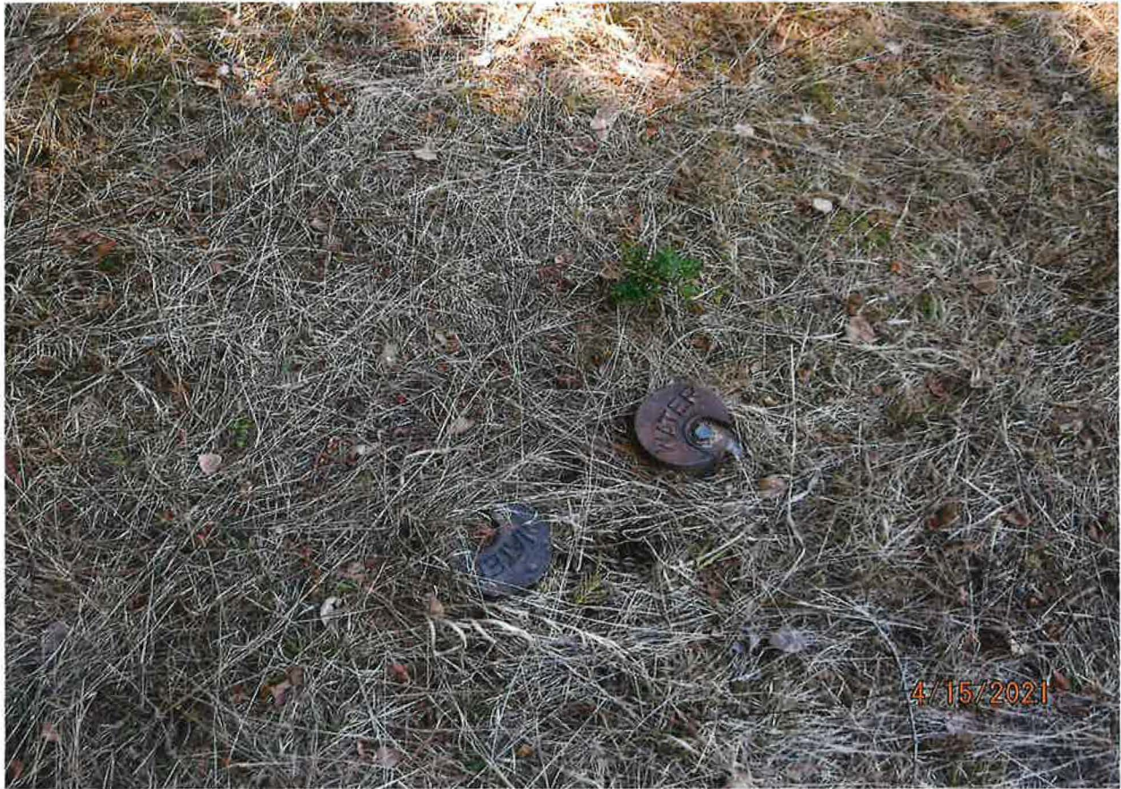
WATER MAIN LINE FROM STORAGE RESERVOIR TO PUMP STATION UTILITY DOME
