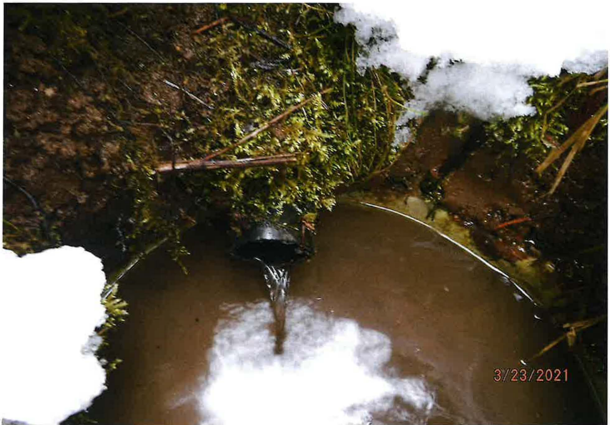
OVERFLOW DISCHARGE FROM POD CULVERT, FLOWS DOWNGRADE INTO CREEK
