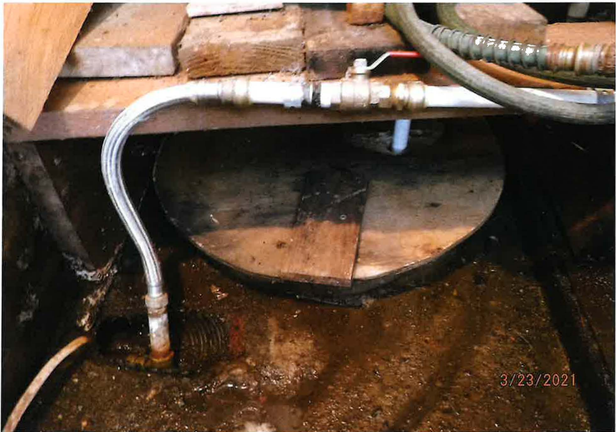
SMALL CISTERN FILLED BY EITHER SPRING WATER (87-10573) OR GNAT CREEK WATER BY FAUCET VALVE
