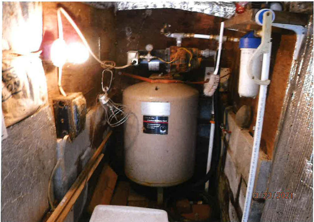
WATER FROM CISTERN ROUTED TO POU VIA PRESSURE TANK AND POLY PIPE
