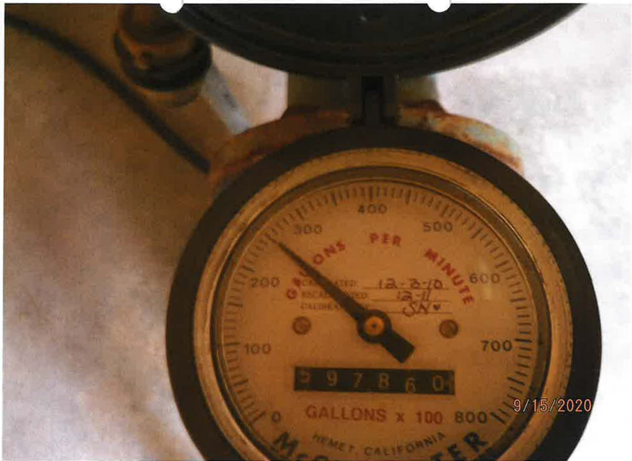
WELL No. 1 – 60 HP PUMP WITH 250 GPM FLOW RATE
