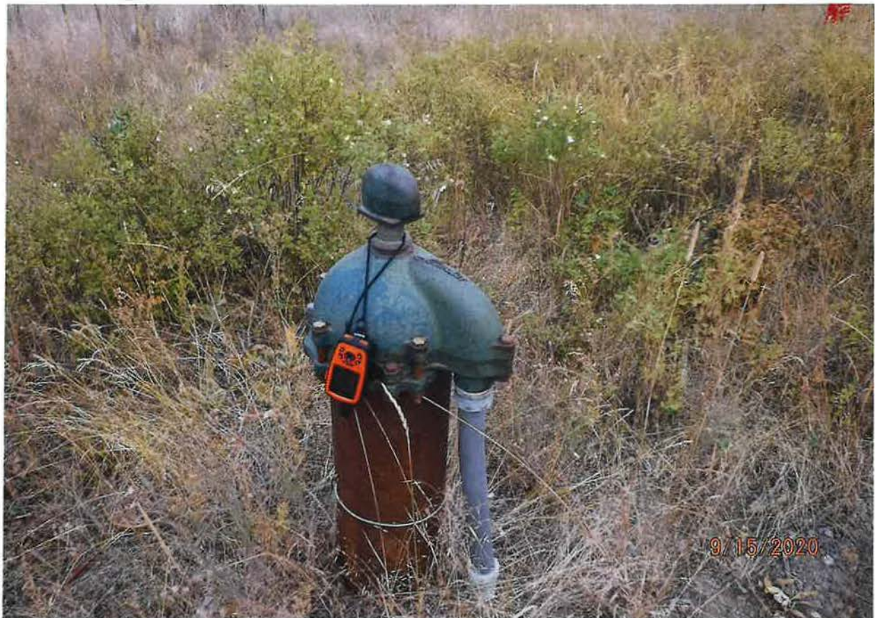
POD - WELL No. 1 95-86-N-125
