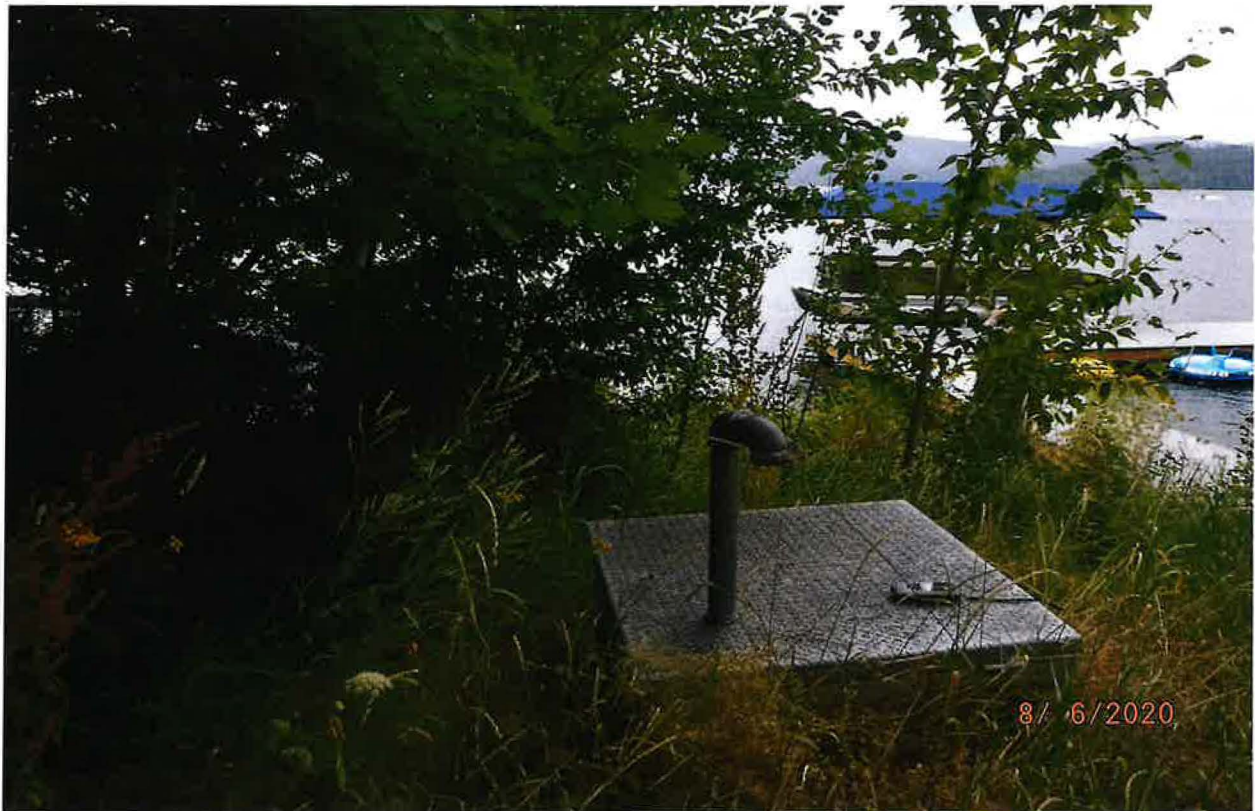
2EA INTAKE PIPES ENTER VAULTED MANIFOLD AND COMMON PIPE LINE TO SLOW SAND FILTRATION PLANT OPERATION
