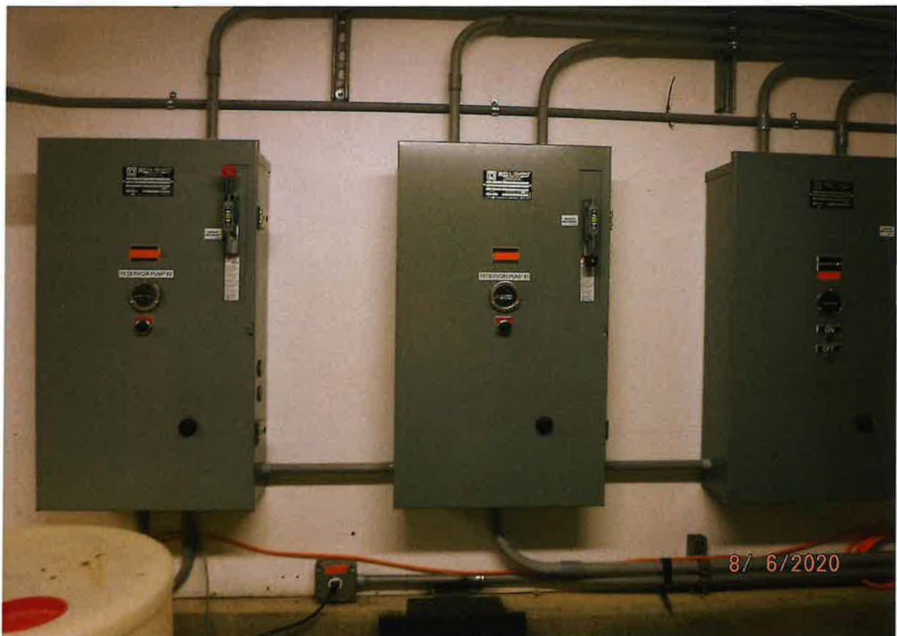
PUMP CONTROL PANELS
