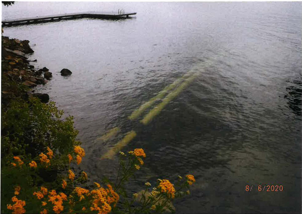
POD – INTAKE PIPES AT SHORELINE
