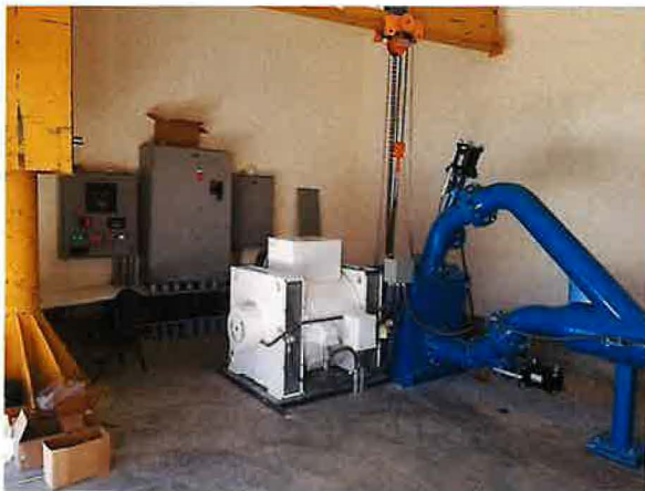
Two Nozzle Pelton Hydro Turbine Generator
