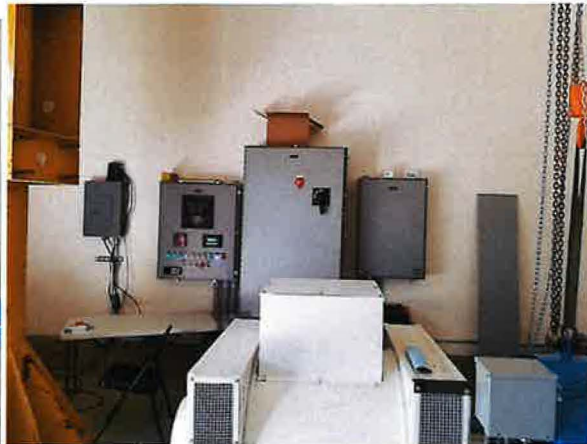
Wall Mounted Hydro Turbine Switchgear and Control Panels
