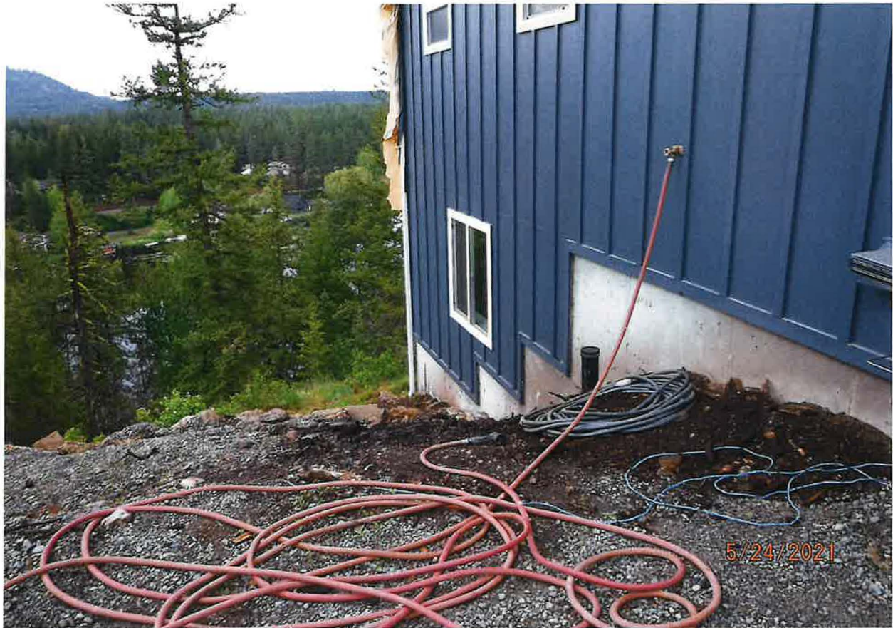
HOSE BIB TO GARDEN HOSE AND SPRINKLER FOR EXTERNAL DOMESTIC IRRIGATION USE
