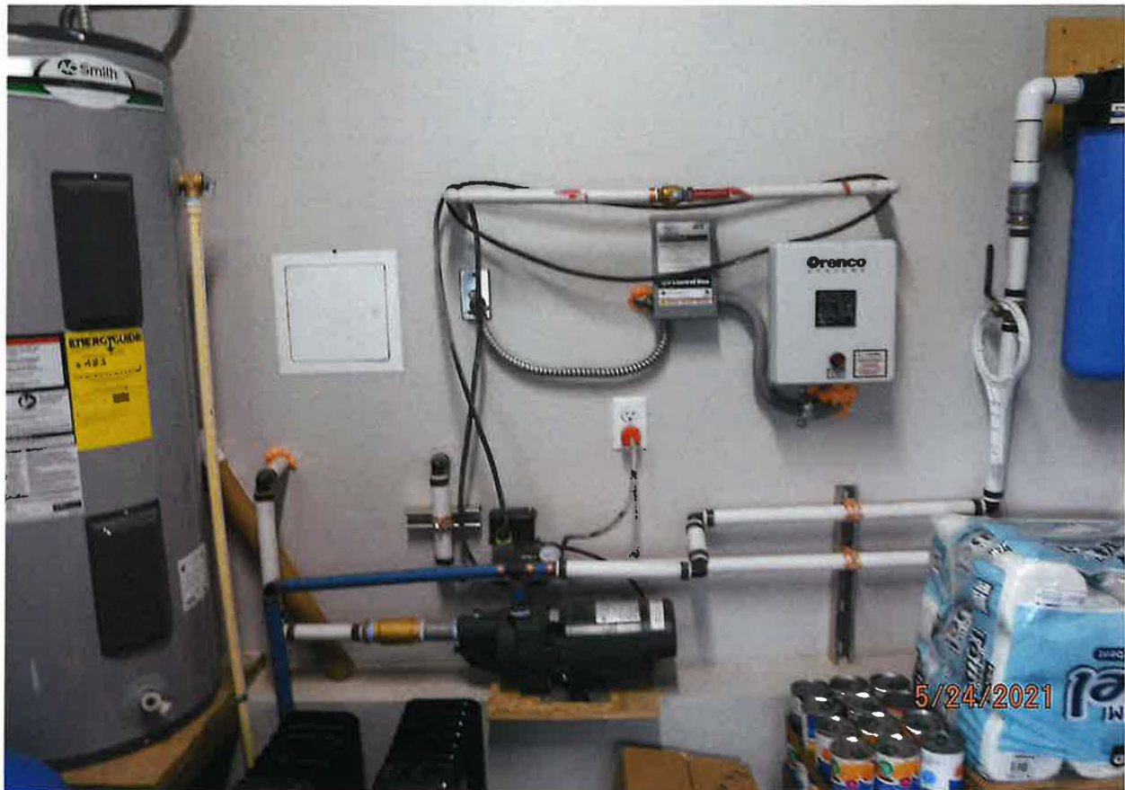
WATER CONVEYANCE SYSTEM – SET UP IN GARAGE NEXT TO RESIDENCE
