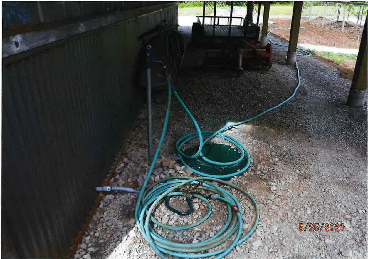
3 EA FROST FREE HYDRANTS INSTALLED IN SYSTEM, WITH 6 LB PRESSURE TANK (VAULTED IN IMAGE)
