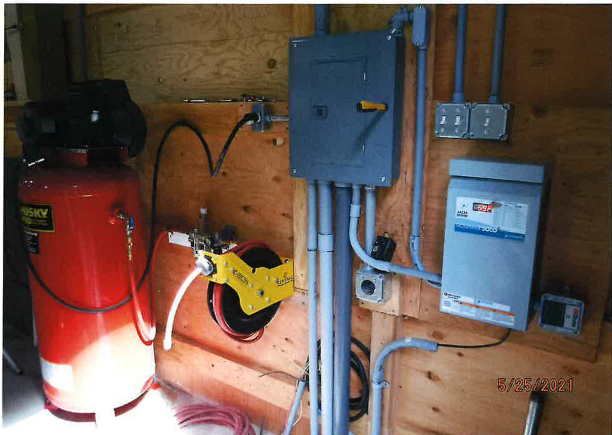
IRRIGATION SYSTEM CONTROL PANEL
