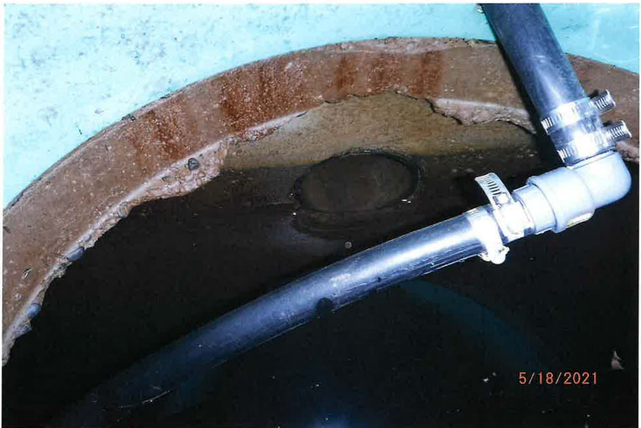
24 HR IMPOUNDMENT TANK – INFLOW PIPE; BLACK POLY IS RETURN LINE FROM SPRINKLER SYSTEM ALLOWING SELF DRAIN AFTER EACH SYSTEM OPERATION
