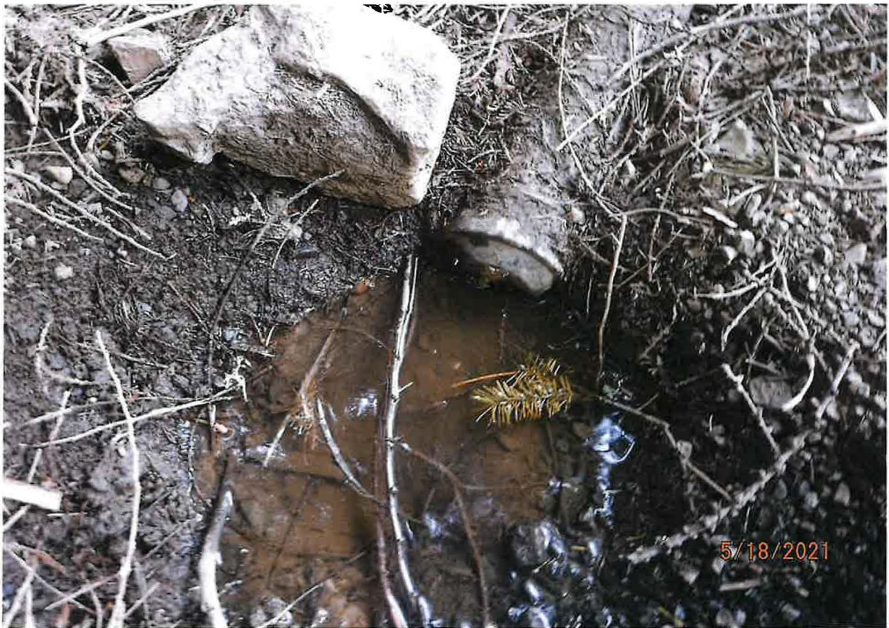
AT POD – SPRING WATER ENTERS PIPE TO 24 HR IMPOUNDMENT TANK
