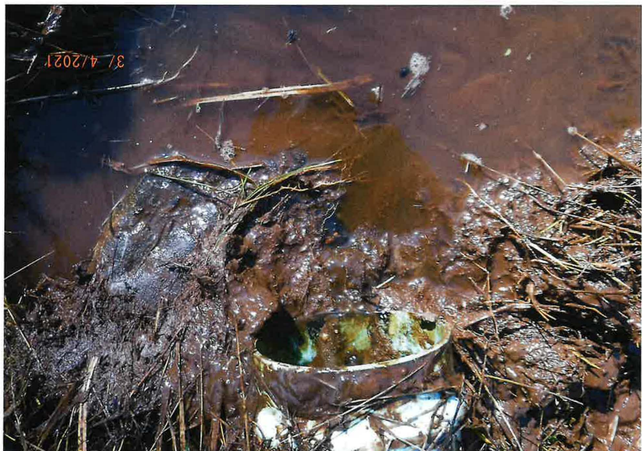
PVC PIPE FROM SPRING BOX ENTERING POND 2 – MINIMAL FLOW < 0.01 CFS OBSERVED
