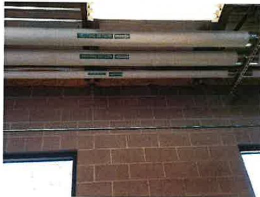
Piping for the heating/cooling system
