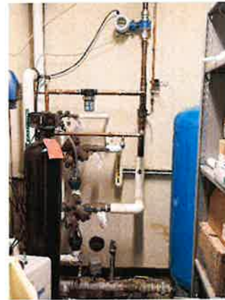
Vales, pressure tank, and chlorination for domestic water inside the facility
