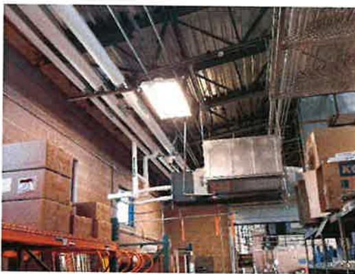
Heating/cooling piping and equipment
