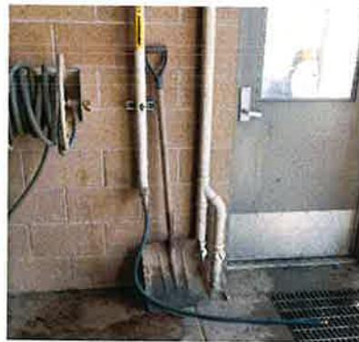
One of the hose bibs inside the shop used for vehicle washing
