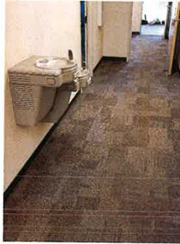
Drinking water fountain outside of men's and women's restroom inside the office building
