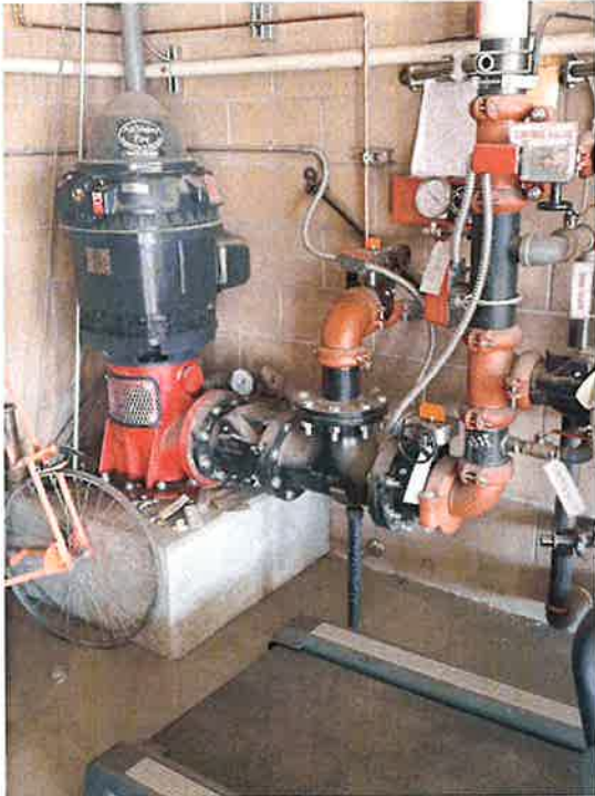
Fire pump, valves, and piping
