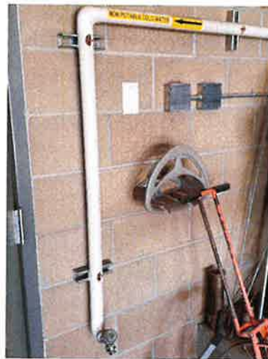
One of the hose bibs inside the shop used for vehicle washing
