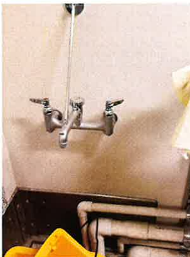
Sink inside room with domestic water valves and pressure tank
