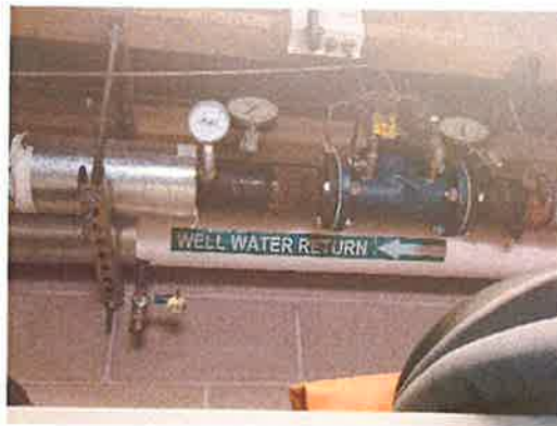
Piping and valve for the heating/cooling system
