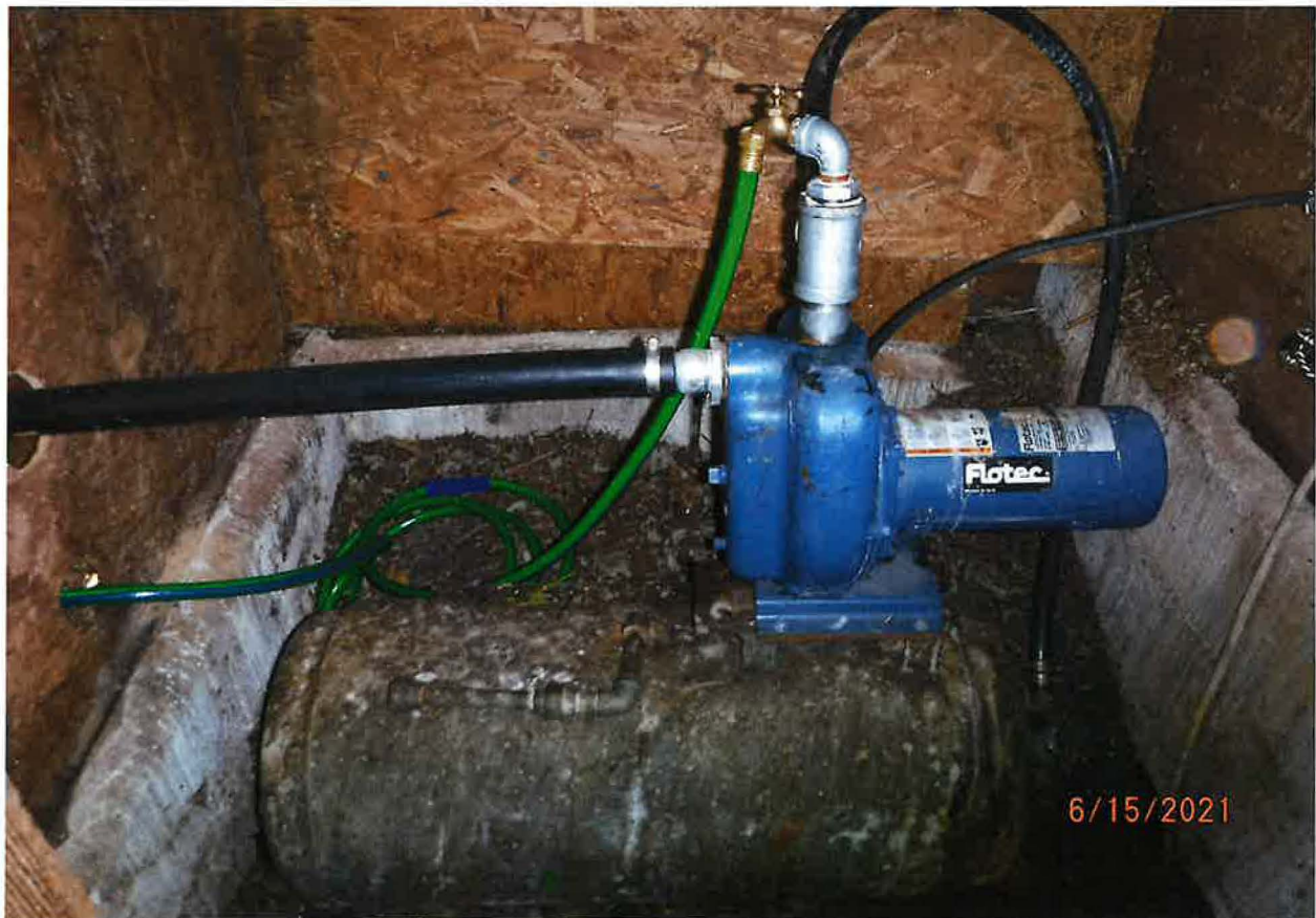
FLOWTEC 1.5 HP WATER TRANSFER PUMP INSTALLED
