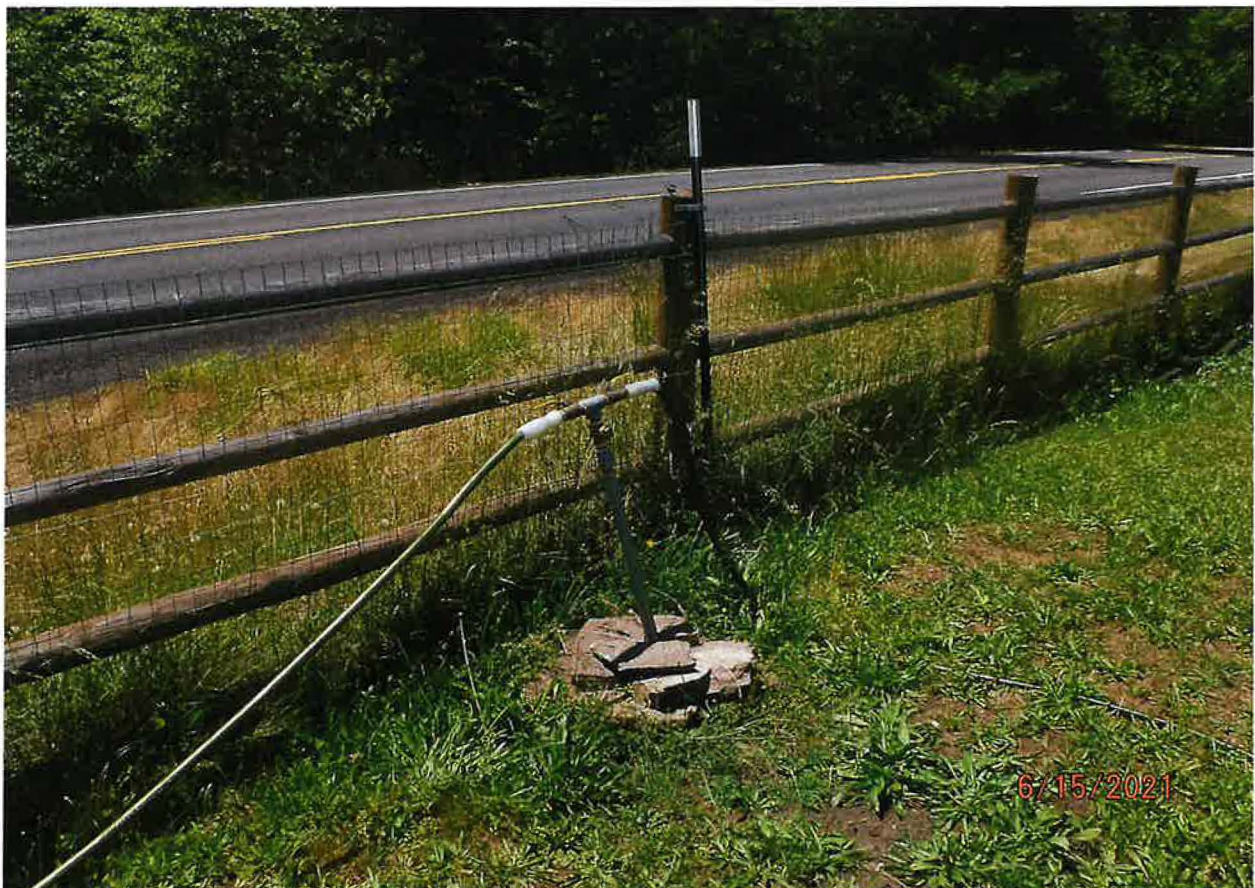
WATER LINE TO IRRIGATION RISER PIPE – OPERATES 2 EA HOSE-TO-TRIPOD SPRINKLERS
