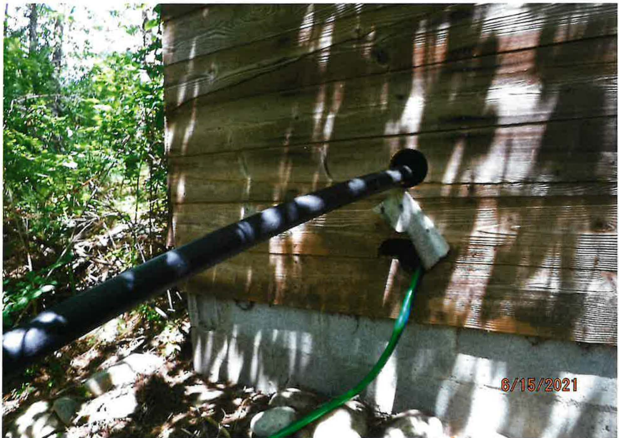
2 INCH POLY PIPE FROM RIVER ROUTED INTO SMALL PUMP HOUSE
