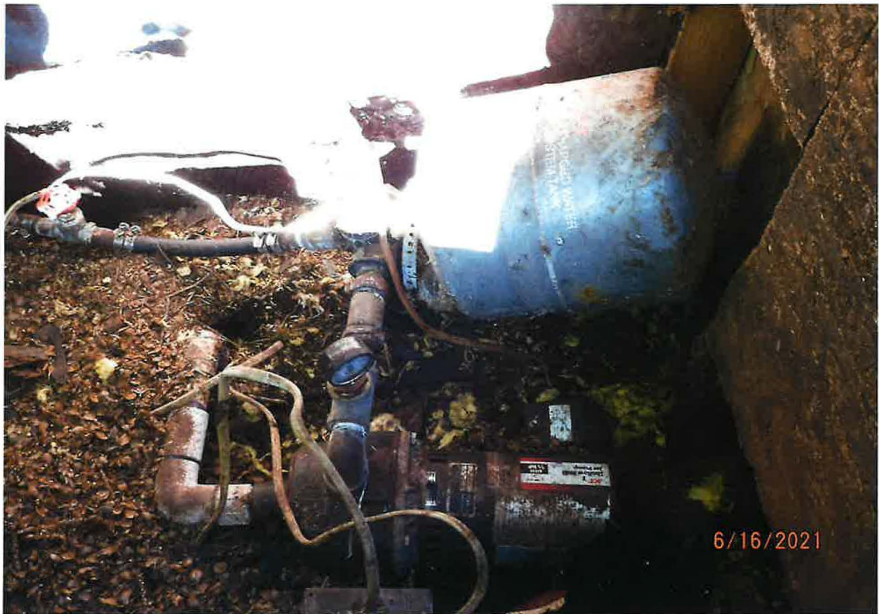
1 INCH PVC PIPE USED TO PUMP FROM CISTERN-TO-PRESSURE POT-TO POLY PIPE SERVICE LINE
