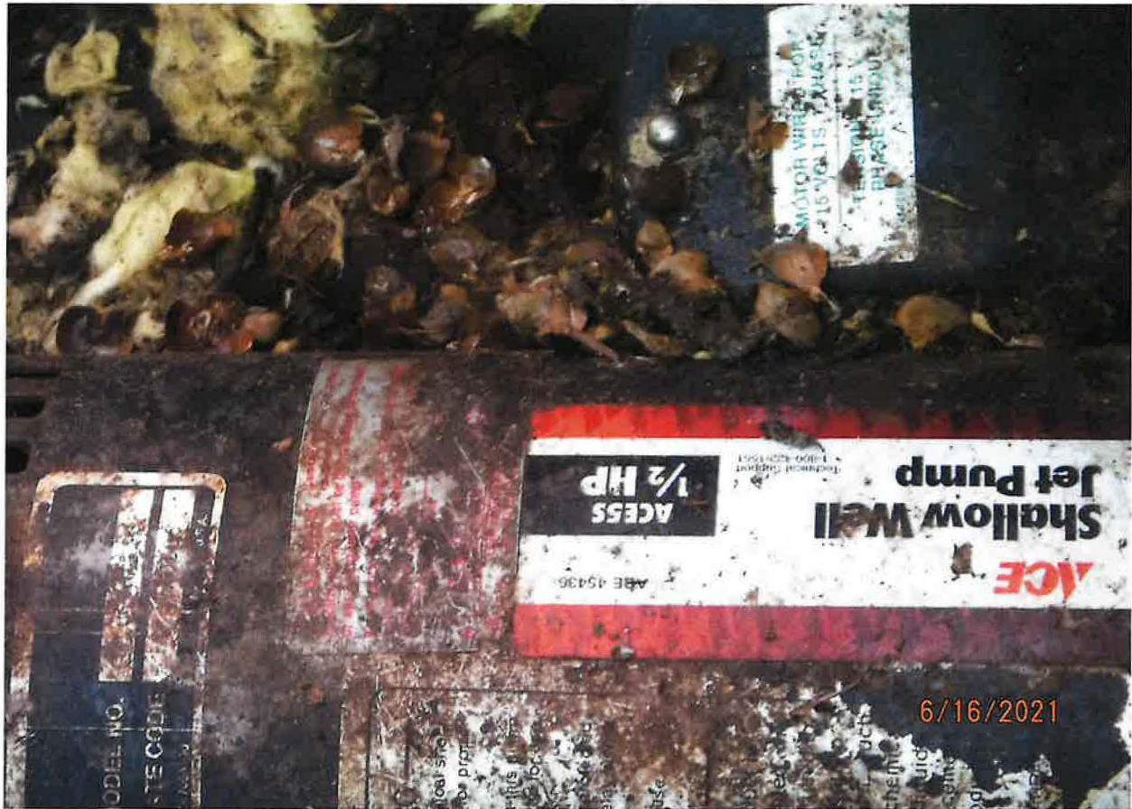
1/2 HP PUMP INSTALLED IN DIVERSION SYSTEM
