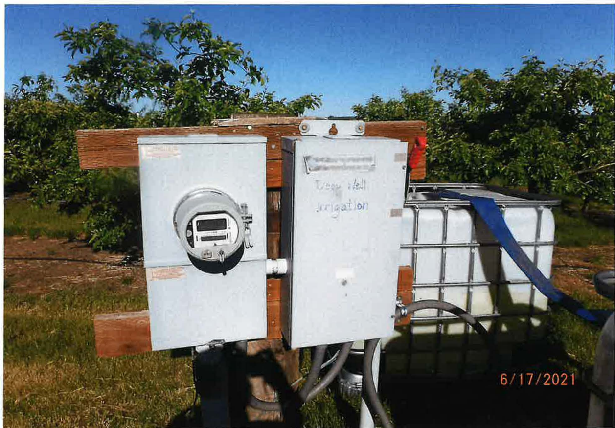
PUMP CONTROL PANEL – 20HP PUMP INSTALLED IN WELL
