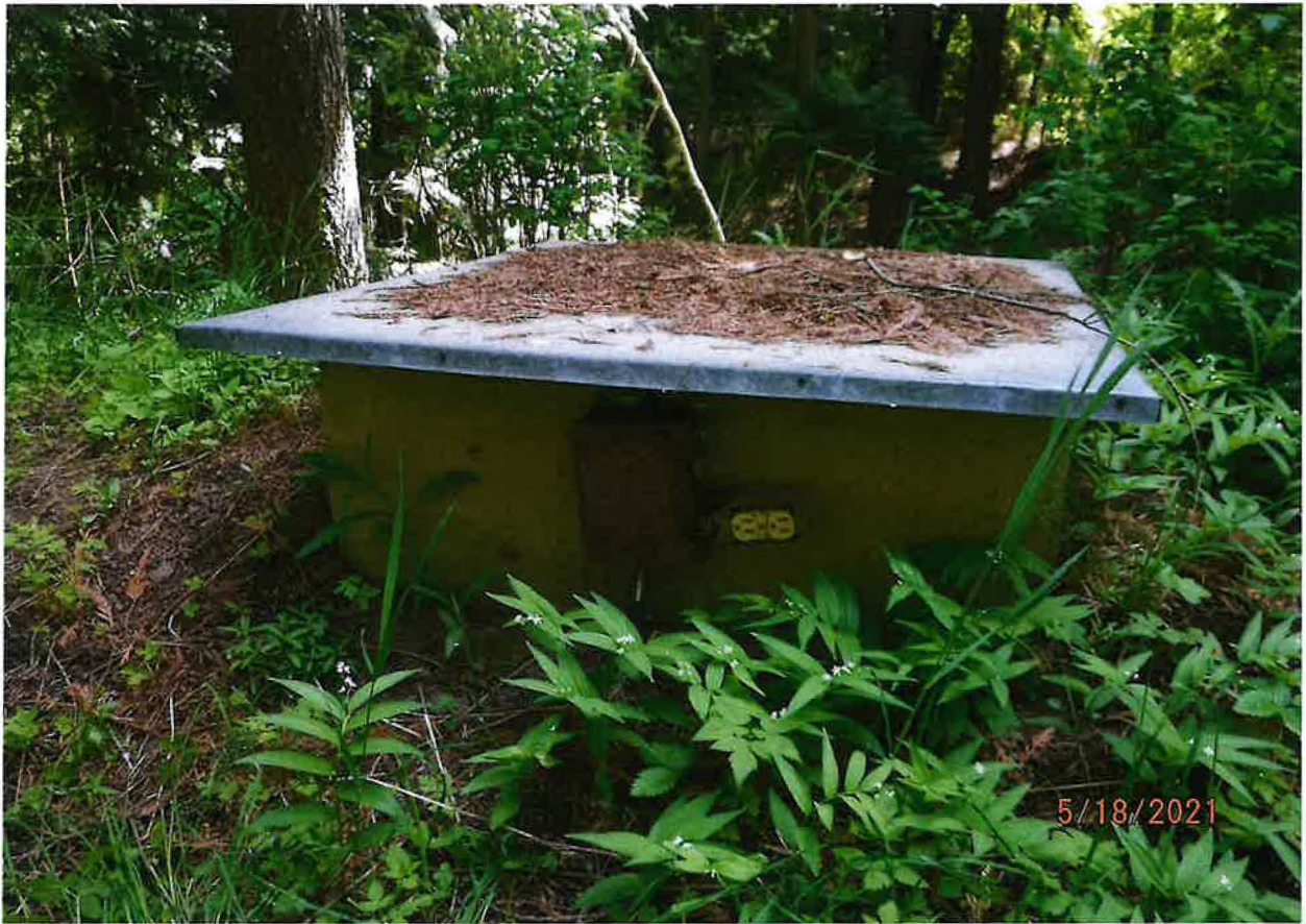
WATER PUMPED FROM RESERVOIR UPHILL (80 FT ELEVATION GAIN) TO PUMP HOUSE
