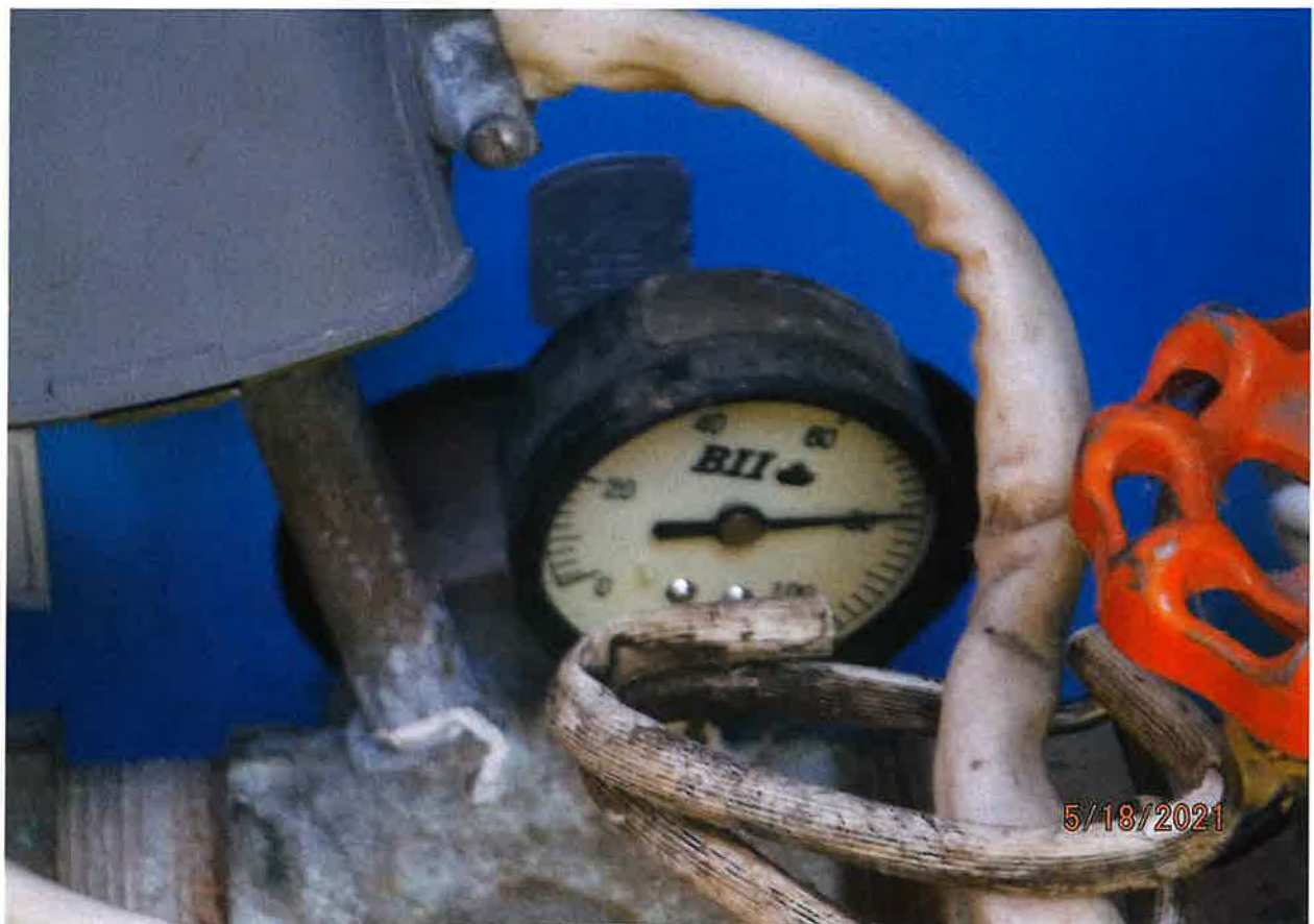
80 PSI SYSTEM OPERATING PRESSURE
