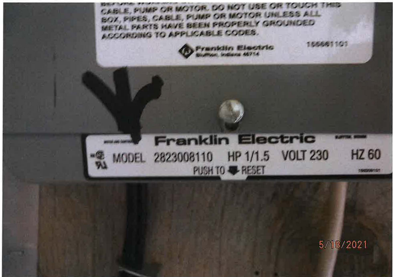
1.5 HP SUBMERSIBLE PUMP INSTALLED ON DIVERTING SYSTEM
