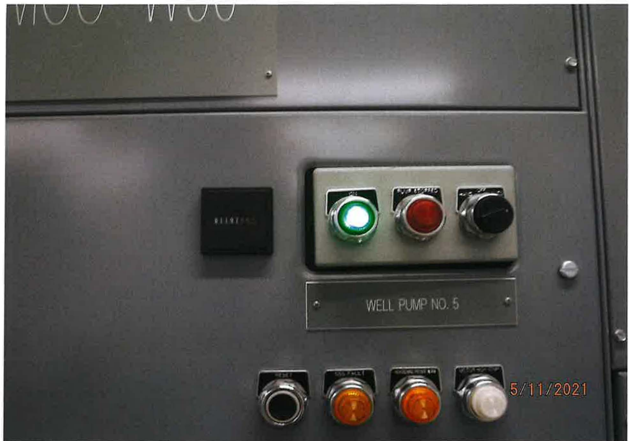
PUMP CONTROL PANEL
