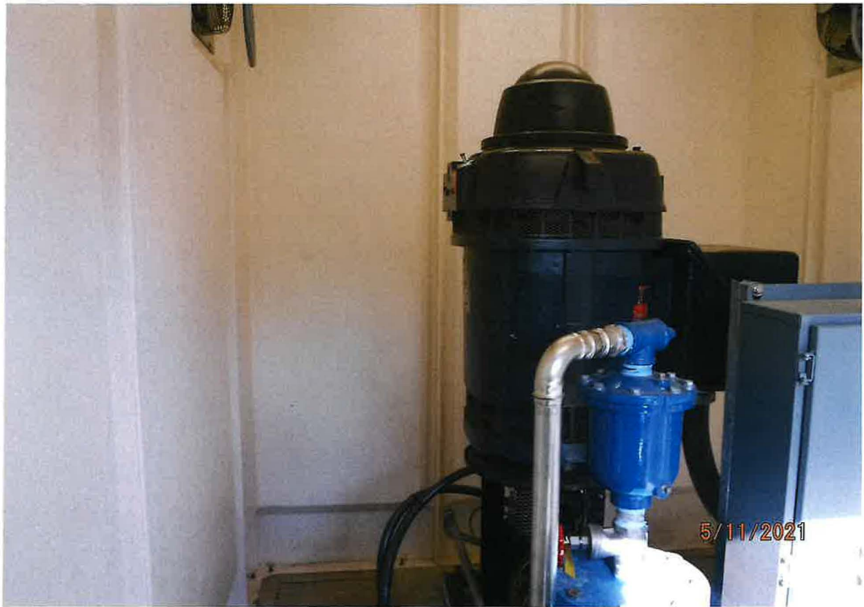
200 HP TURBINE PUMP INSTALLED IN WELL
