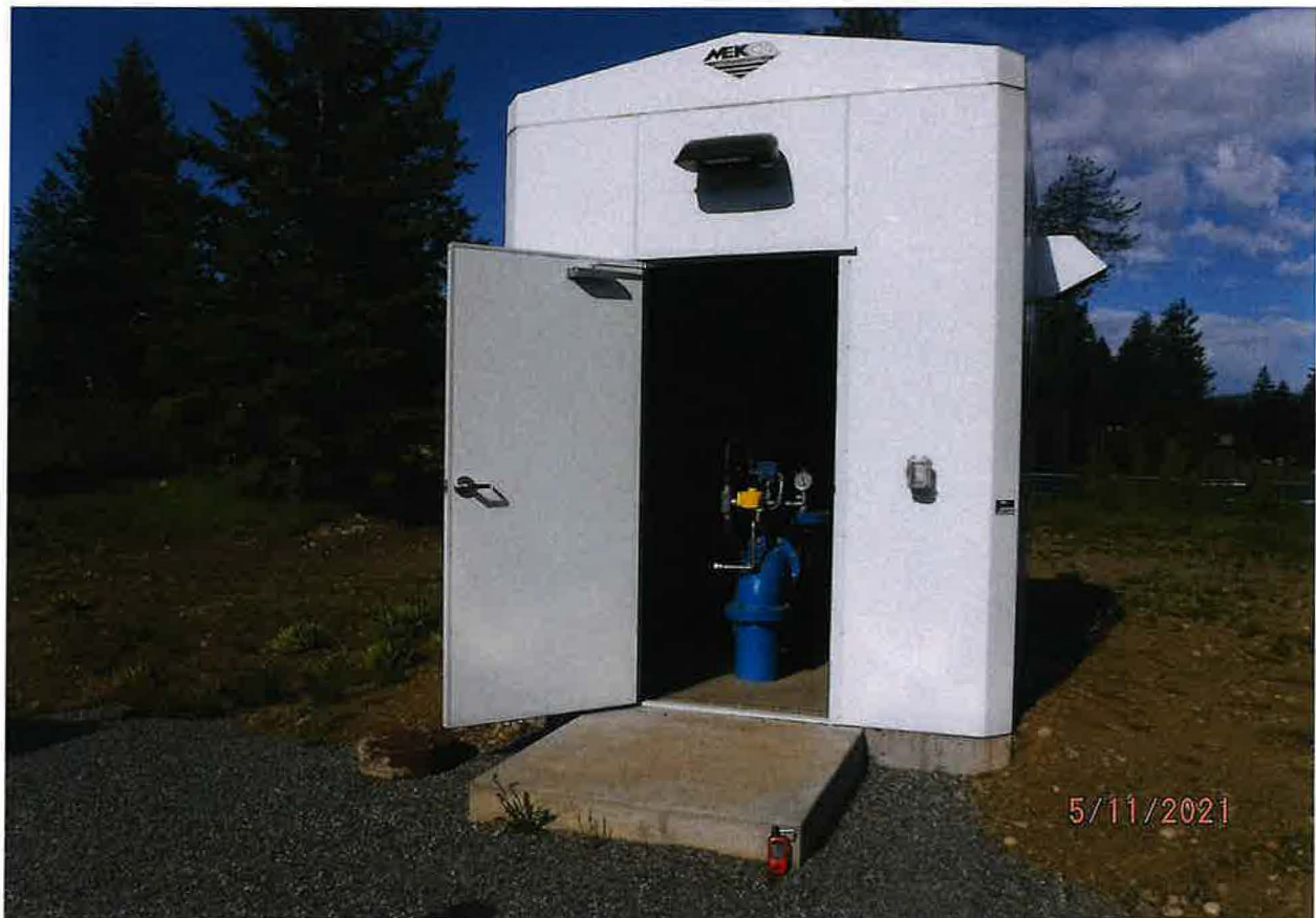
PUMP HOUSE FOR SPIRIT LAKE WELL No. 5
