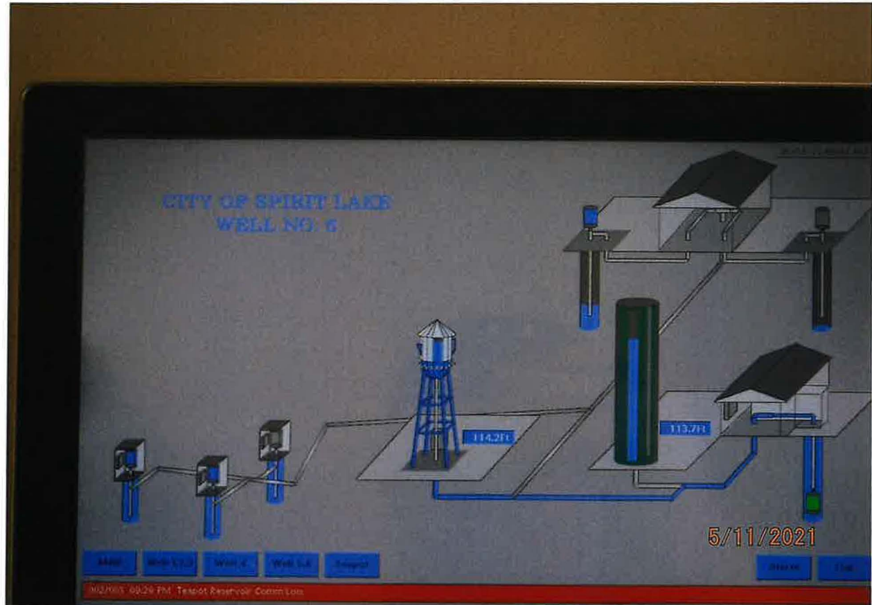
SCADA SYSTEM – MANAGES WELL(S) 1-5
