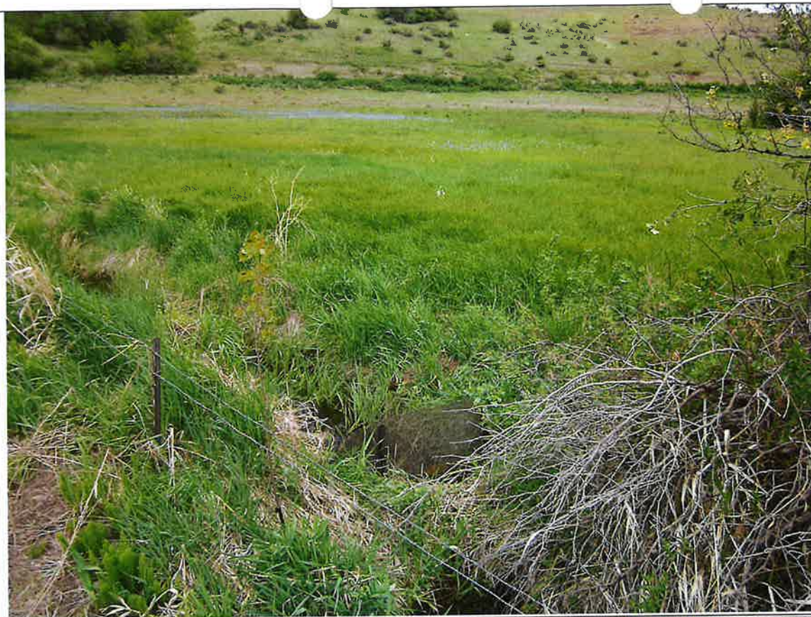
Figure 1. Waste water is collected in a ditch along the property line of northern neighbors property (5/21/2021).
