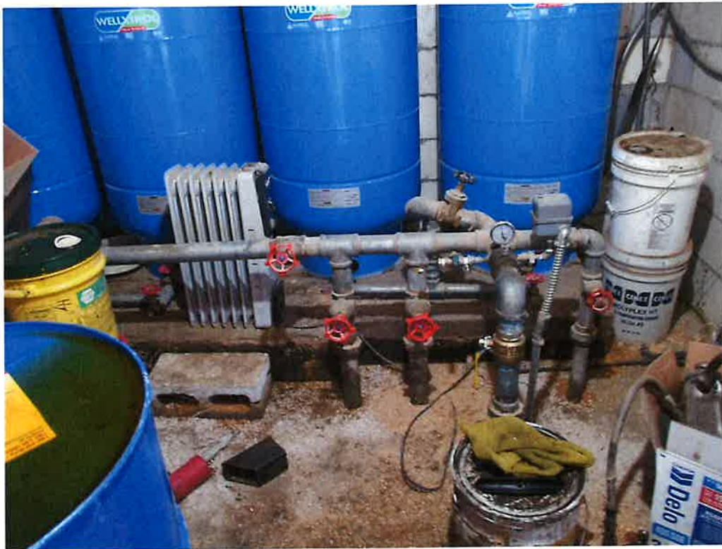
Figure 7 Pump House for Barn Well
