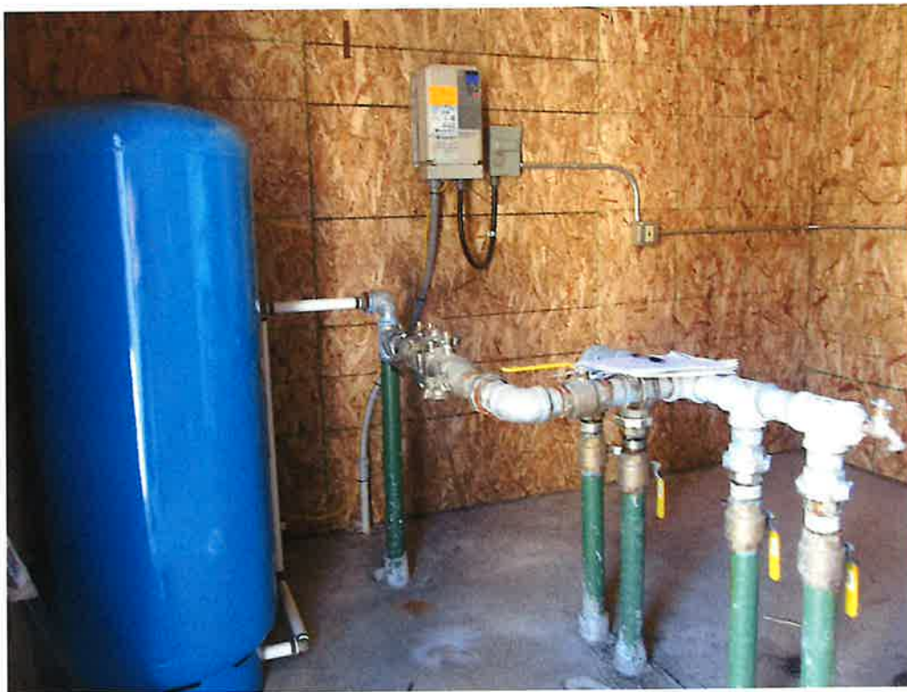
Figure 10 Pump House for the Friday Well
