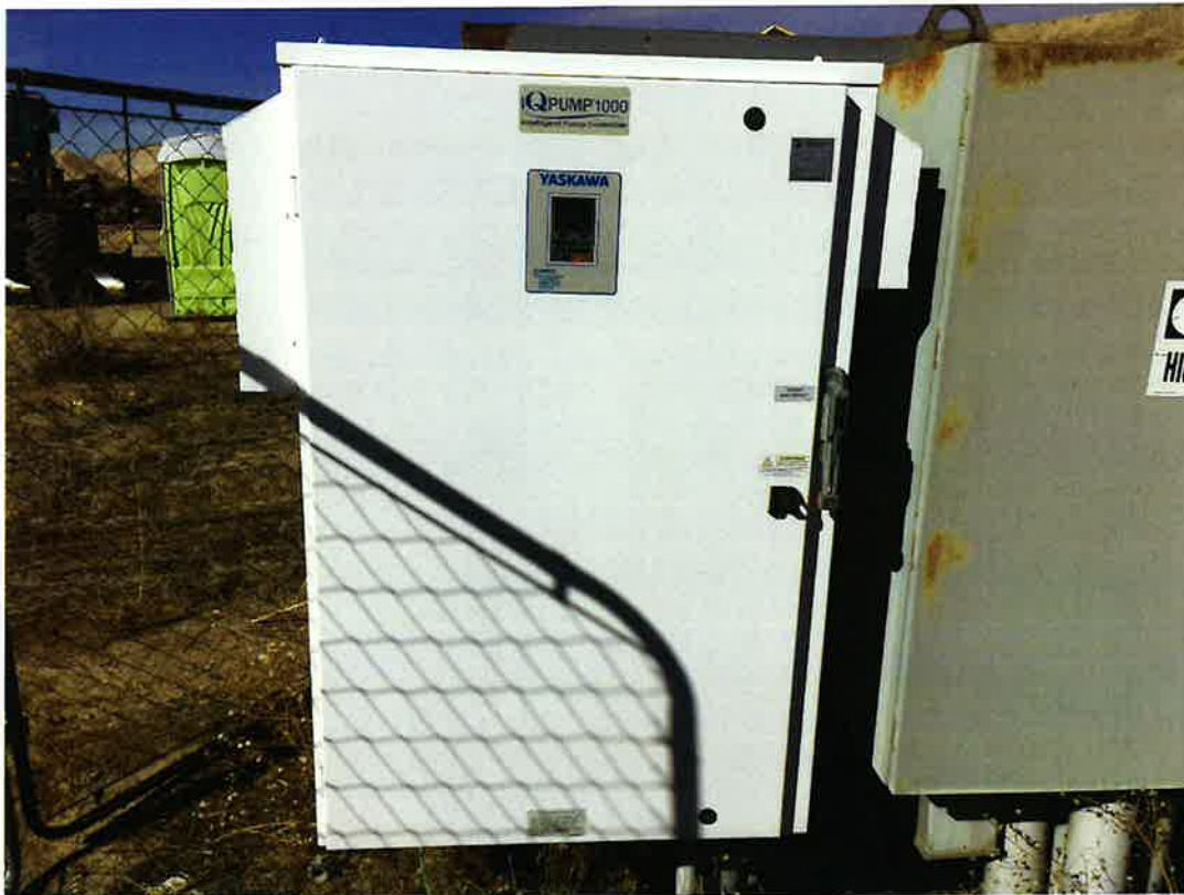
VFD control panel for 50-hp submersible pump
