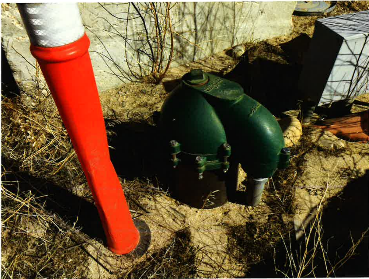
8-inch well head with pitless unit for submersible pump.
