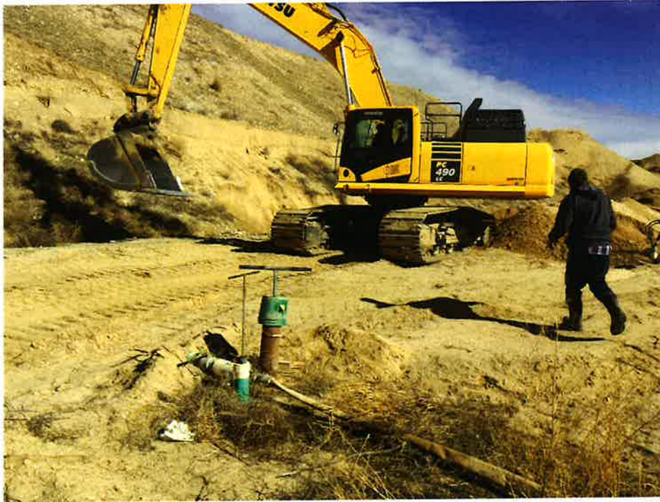
Terminus of pipeline from well. Shut-off valve handles for 4-inch pipeline and for pipeline to yard hydrant.
