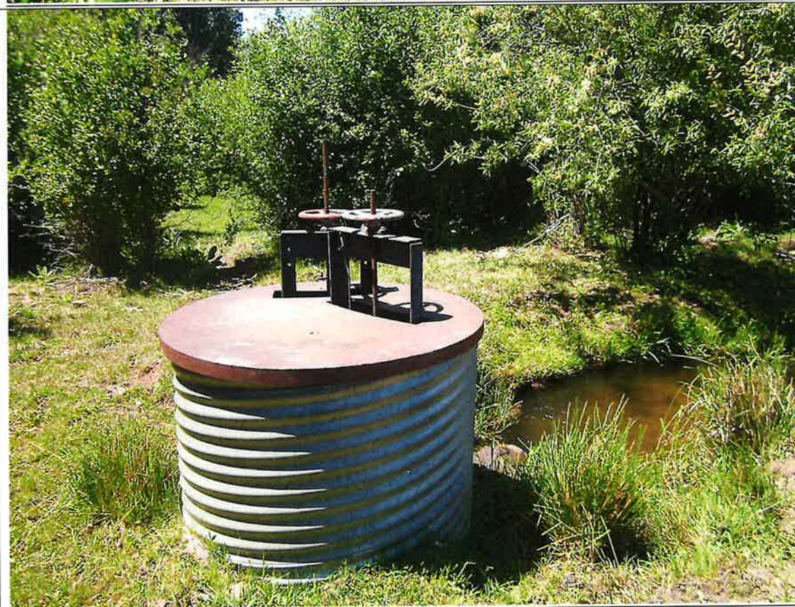
Figure 2. Double gate valves at splitter which diverts water to either north side of creek or south side of creek.
