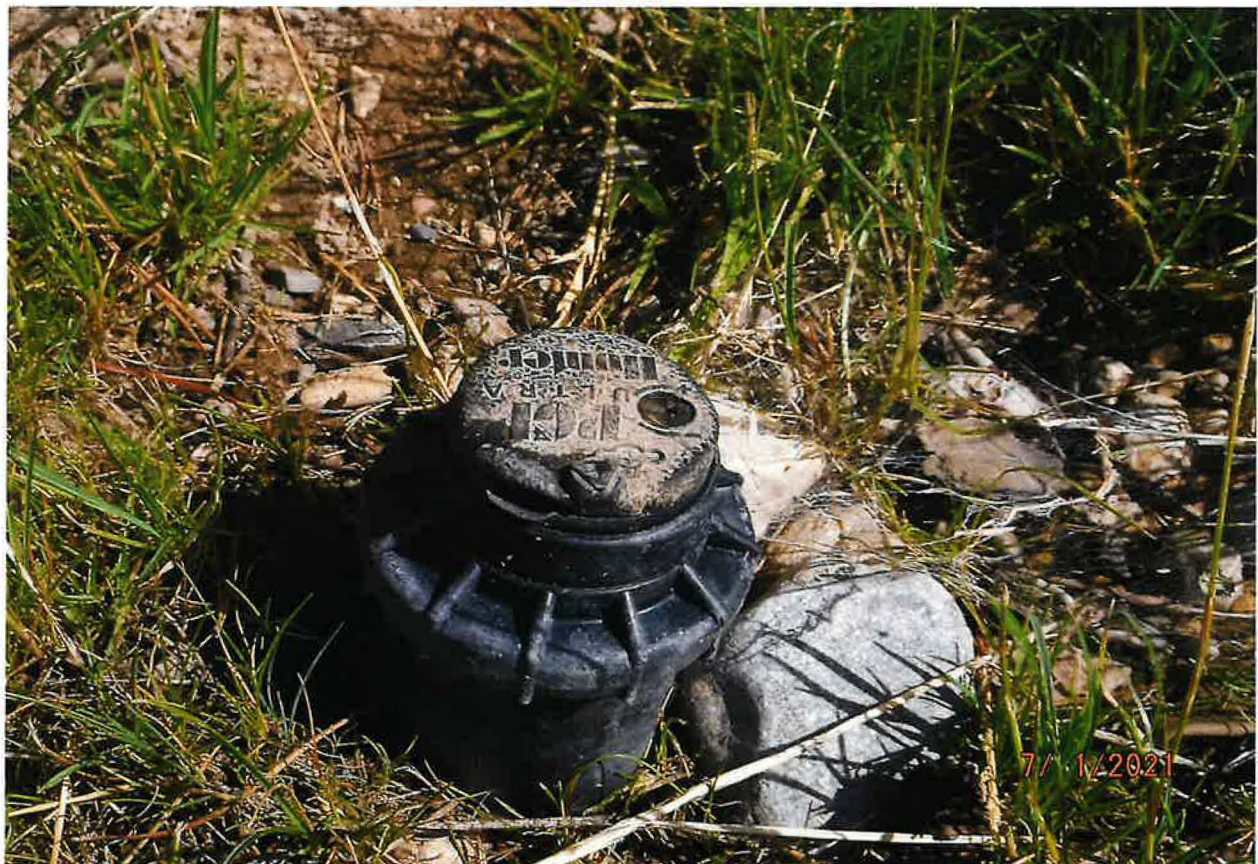
IRRIGATION POU – PRESSURIZED SPRINKLER SYSTEM
