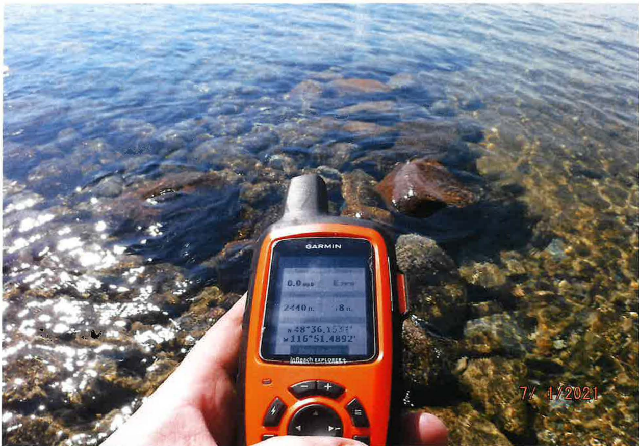
POD – SUBMERGED INTAKE PIPE W/PUMP IN PRIEST LAKE
