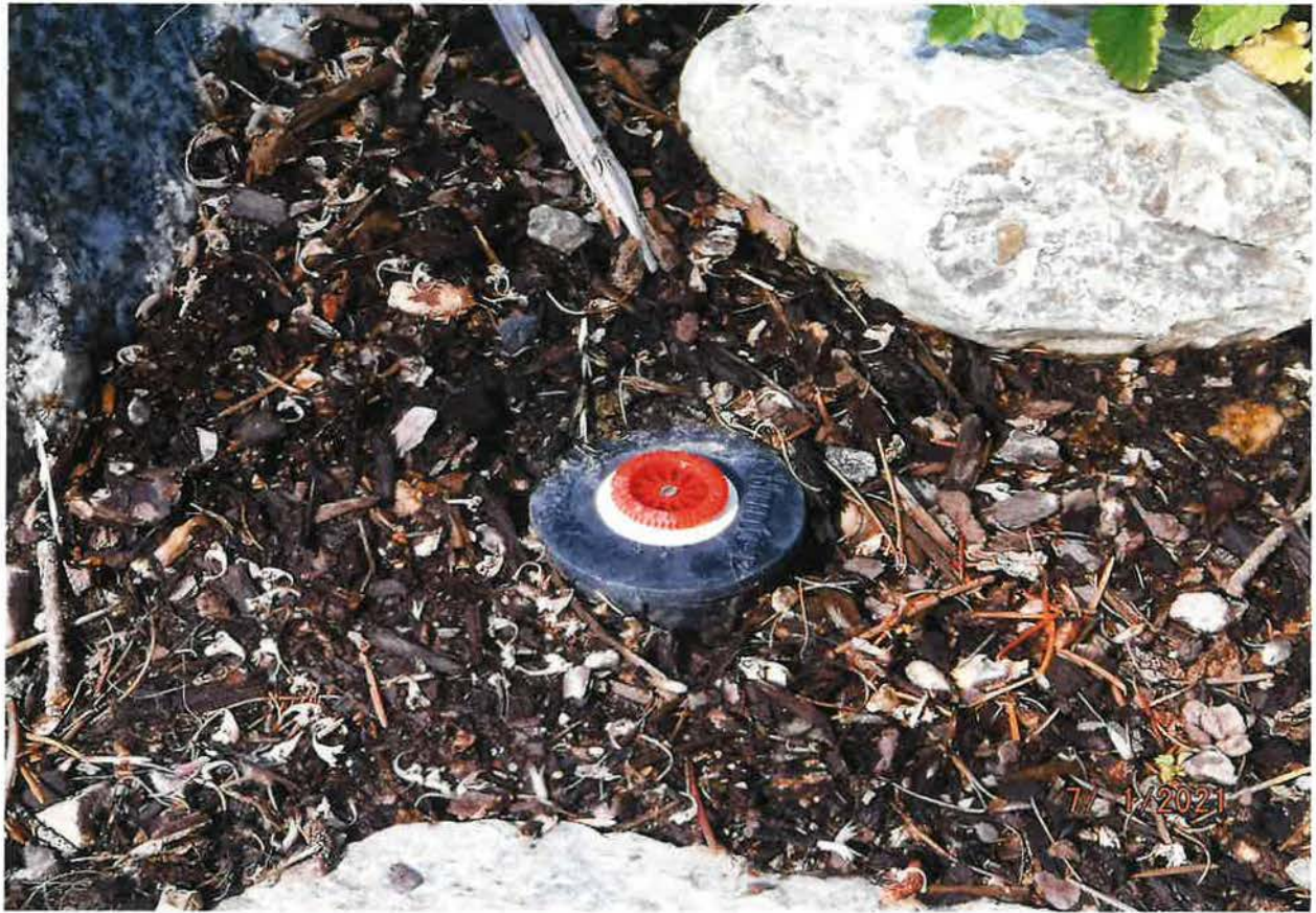
IRRIGATION POU – PRESSURIZED SPRINKLER SYSTEM
