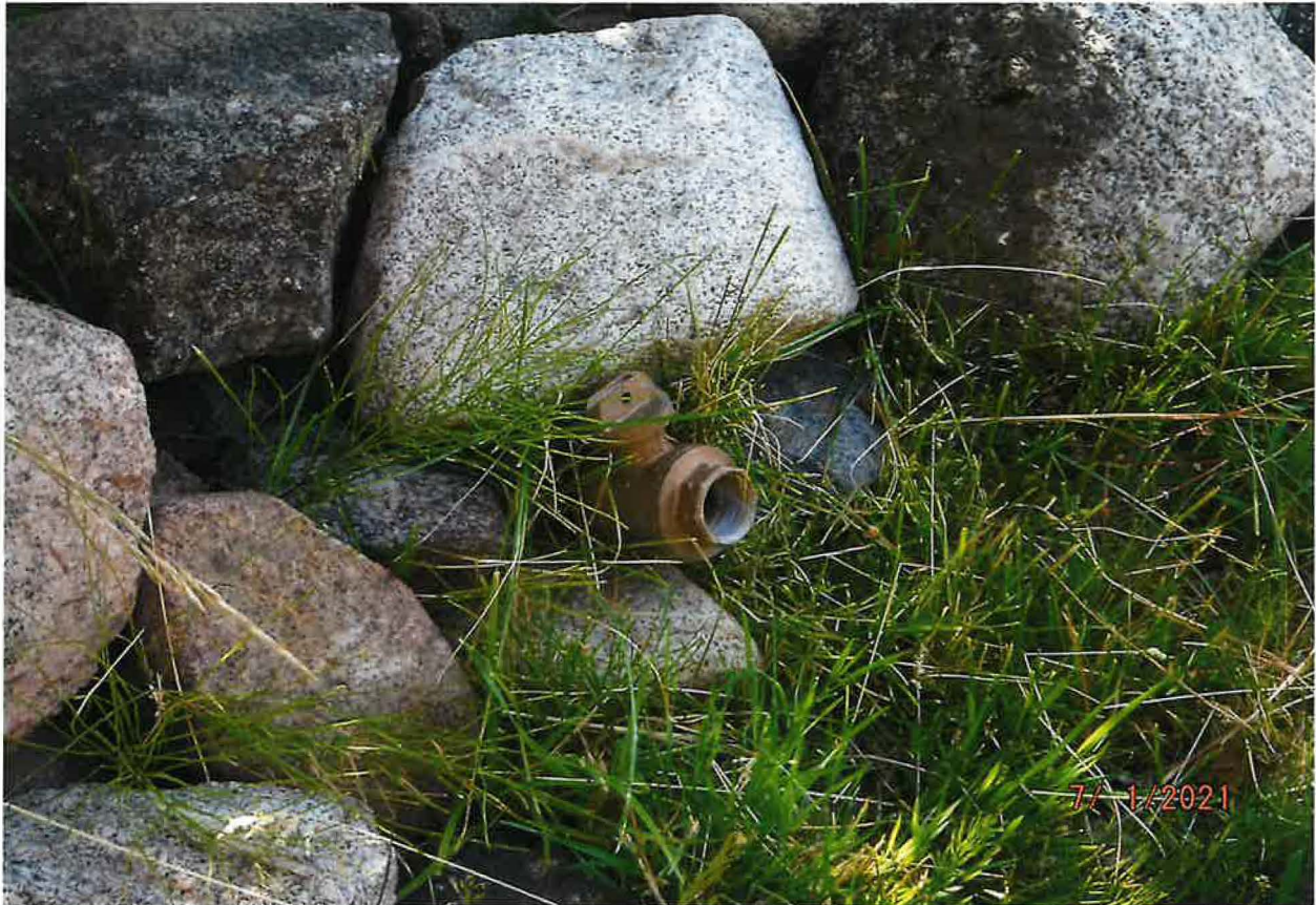
FIRE PROTECTION – 1 OF 2 FIRE HOSE HOOK UP CO-LOCATED WITH POD ALONG SHORELINE
