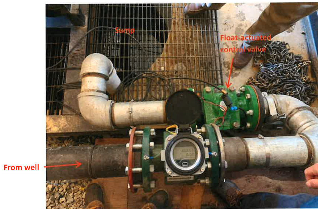
Photo 4: Magnetic flow meter on well inlet line to pump house and vault.
