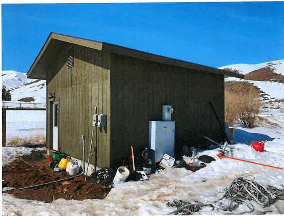
Photo 2: Pump house with storage pond in background, looking west. Well inlet line in red.
