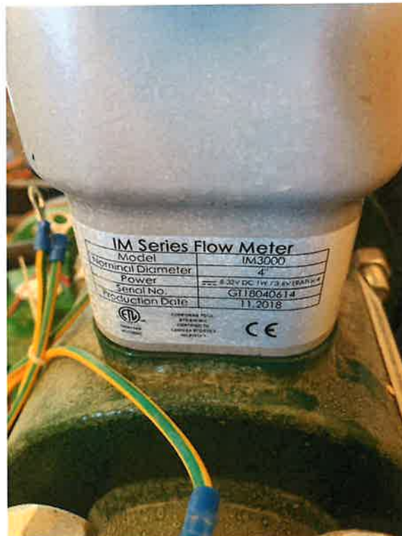
Photo 6: Magnetic meter manufacturer's specifications.
