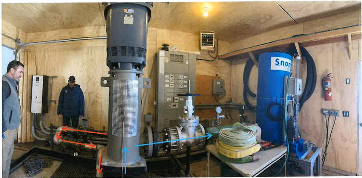
Photo 3: Inside of pump house, line into the pump house in red into sump and pond, blue line is re-pressurized line sending water to snowmaking guns in place of use.
