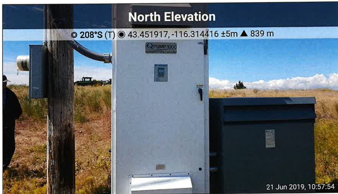
Figure 10: Well 3 variable speed drive controls.
