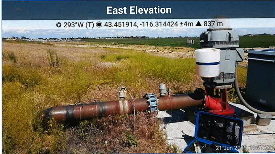
Figure 9: Well 3 equipped with 200-hp motor and vertical turbine pump.
