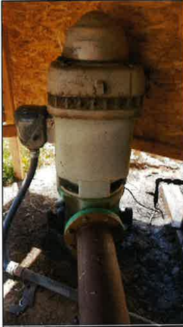
Figure 1: Well 1 75-hp vertical turbine.
