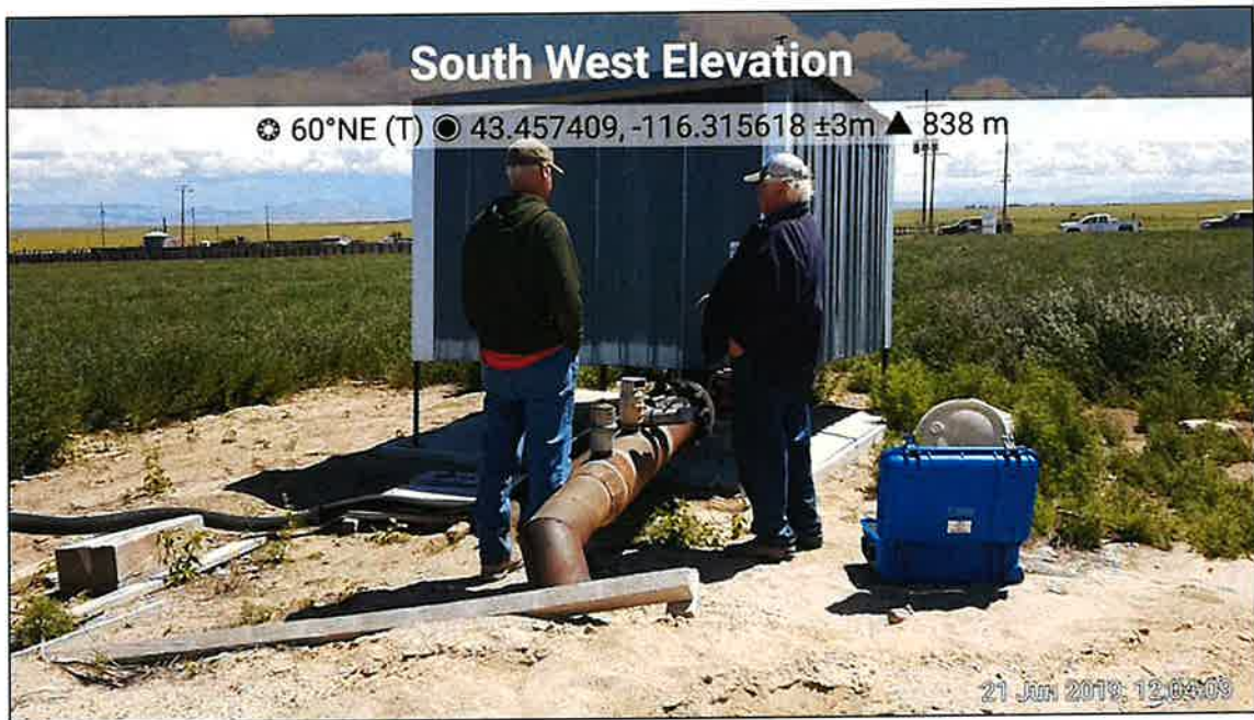
Figure 7: Well 2 equipped with 200 hp motor and vertical turbine pump.
