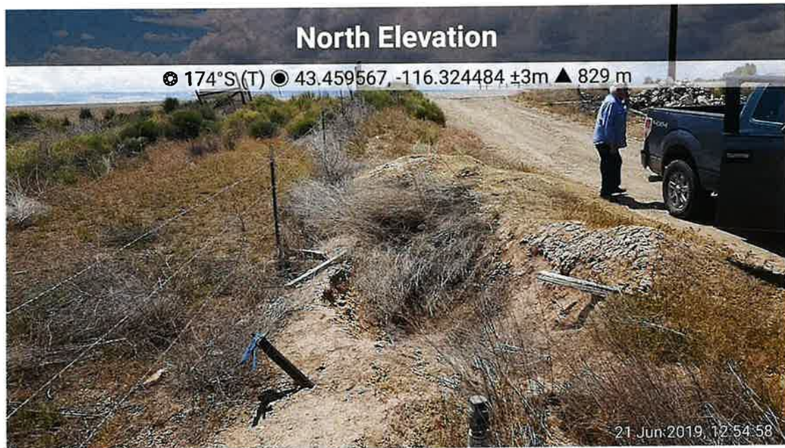
Figure 6: Figure 5 flowmeter installed in pit north of Kuna-Mora Road.
