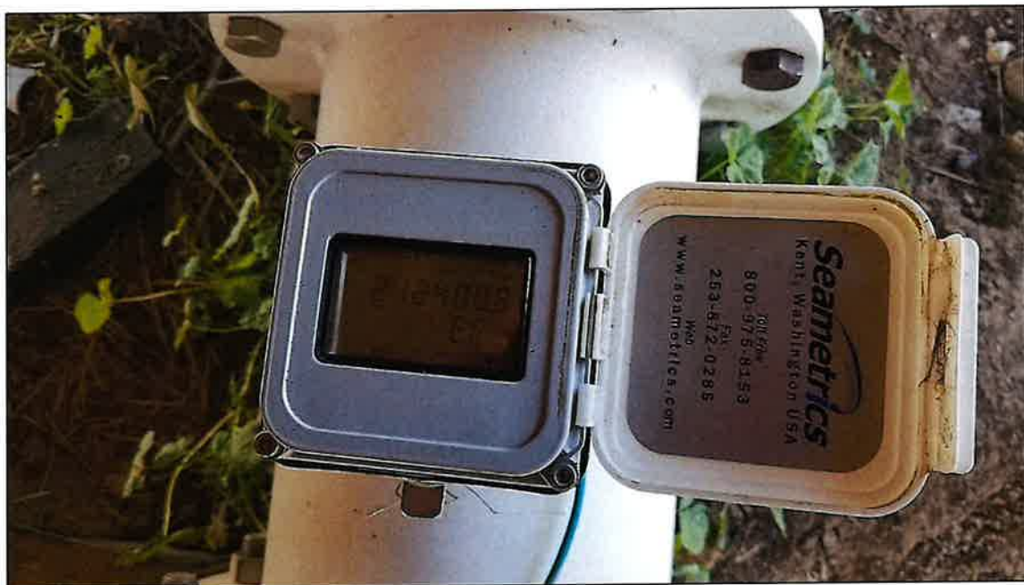
Figure 2: Flowmeter installed on Well 1.
