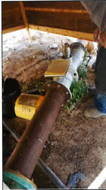
Figure 3: Discharge pipe of Well 1 showing flowmeter location.
