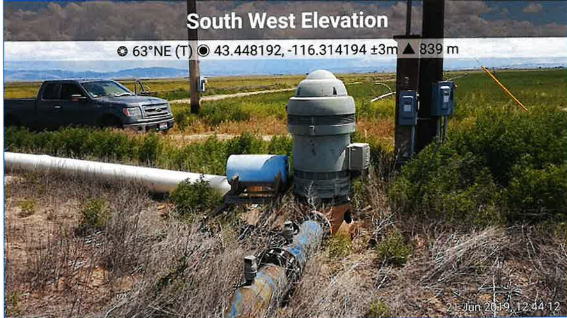
Figure 11: Well 4 equipped with 150 hp motor and vertical turbine pump.
