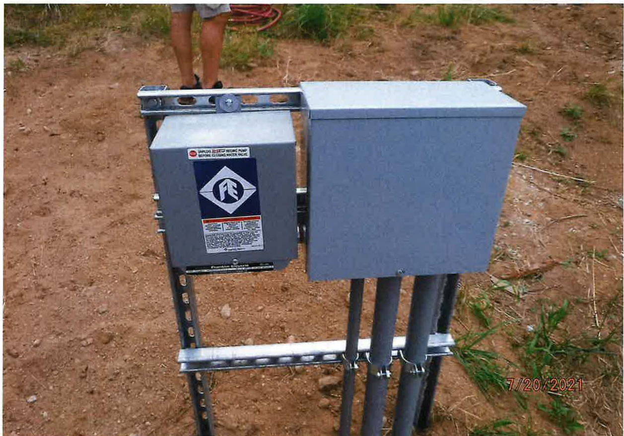
WATER SYSTEM PUMP CONTROL PANEL – LOCATED AT POU
