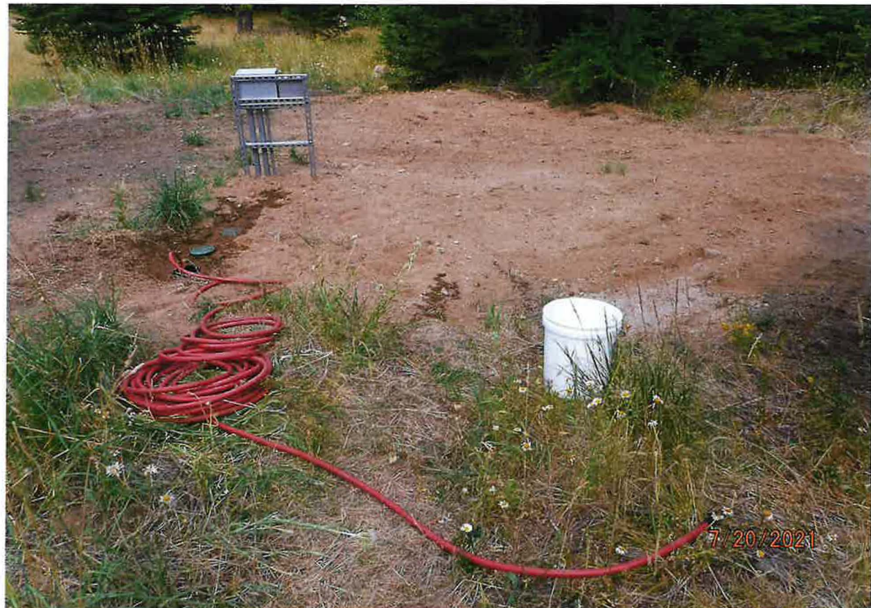
5 GAL BUCKET TESTS COMPLETED FROM INLINE HOSE PORT NEAR PUMP CONTROL PANEL
