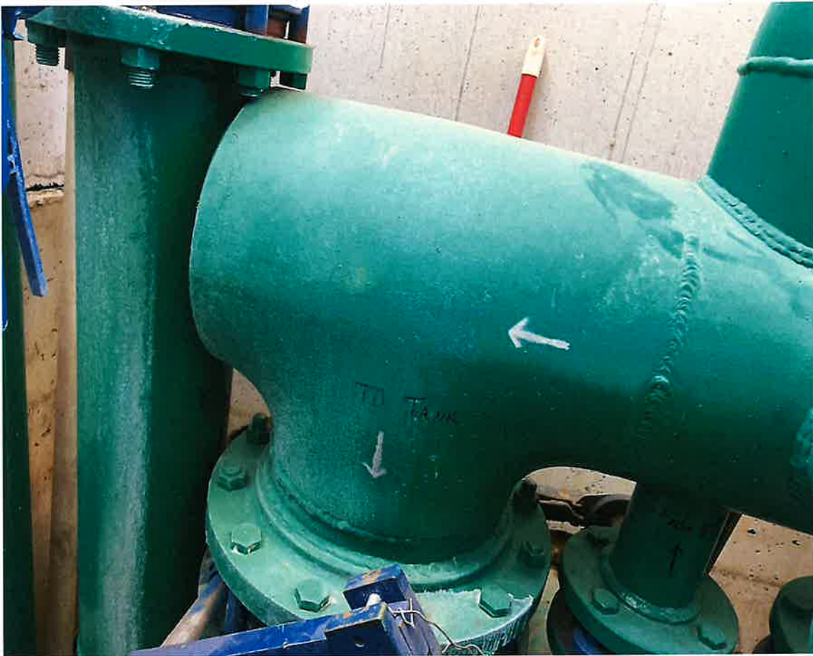
Fig. 13 – Writing indicating flow direction of water in pipes to the storage tanks.
