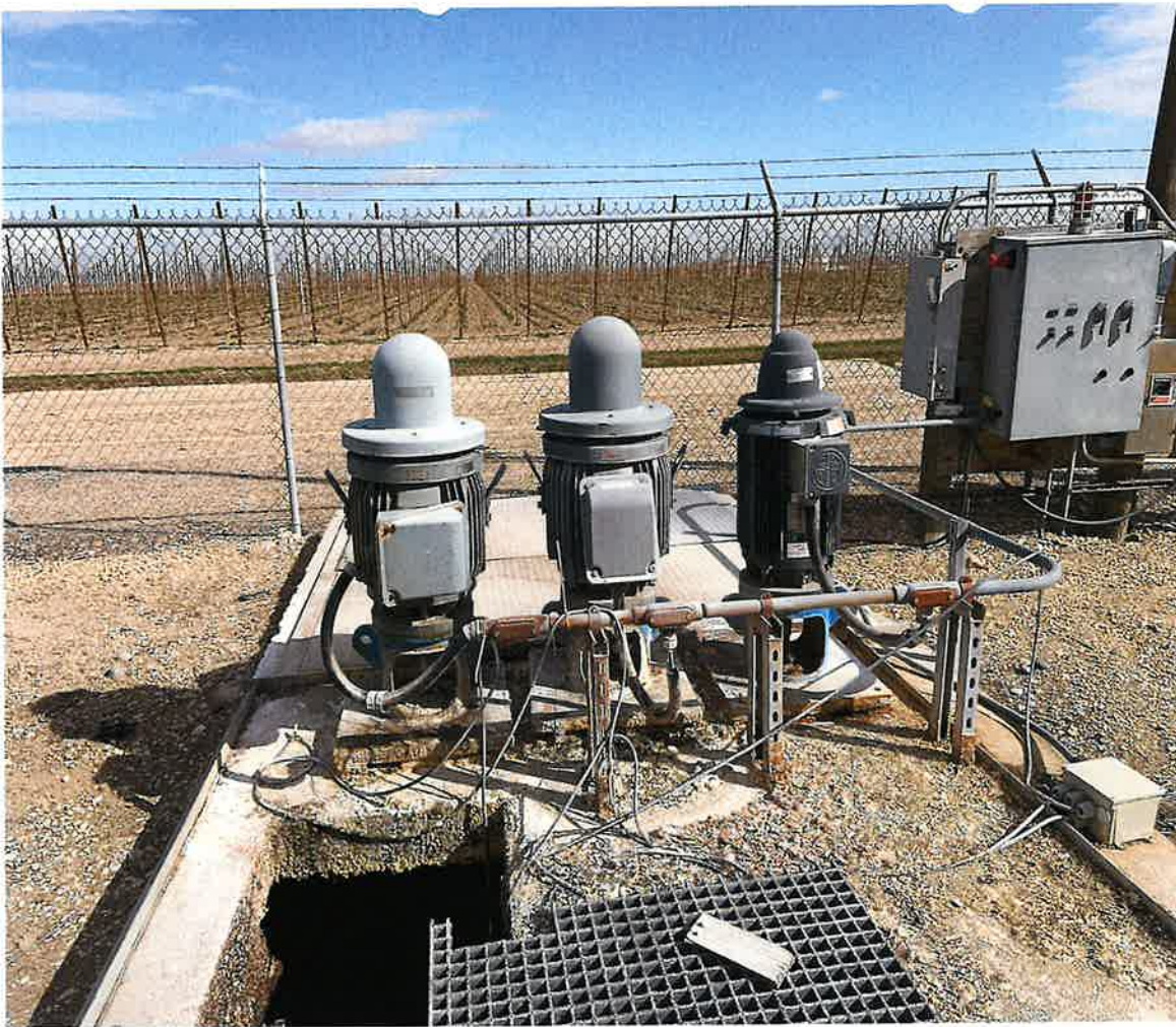
Fig. 19 – Waste water from settling ponds and plant is pumped to the pivot sites using the 3, 25 hp pumps shown.
