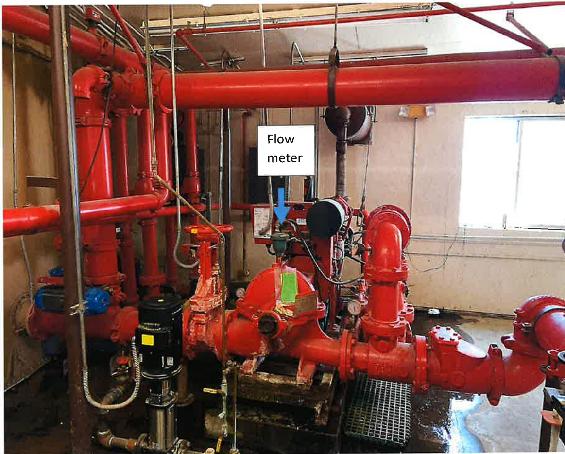
Fig. 17 – Pipes shown are both from wells to eastern tank and outflow from eastern tank to the plant. The flowmeter is also shown.
