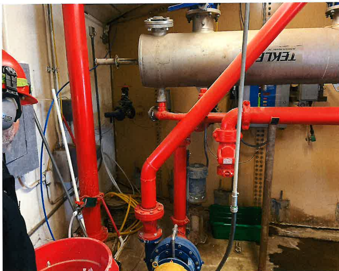
Fig. 16 - View of pipes from eastern storage tank delivering water to the western storage tank. This tank holds chlorinated water used during cleaning of the plant.
