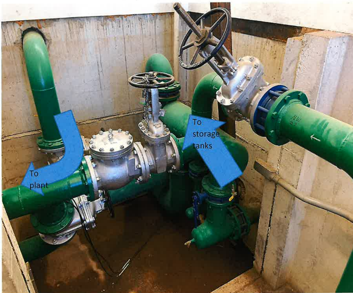
Fig. 9 – Water from the wells comes in from the right side of the picture and goes to the storage tanks. Water comes from the storage tanks via the pipe on the left side of the picture and goes to the plant.
