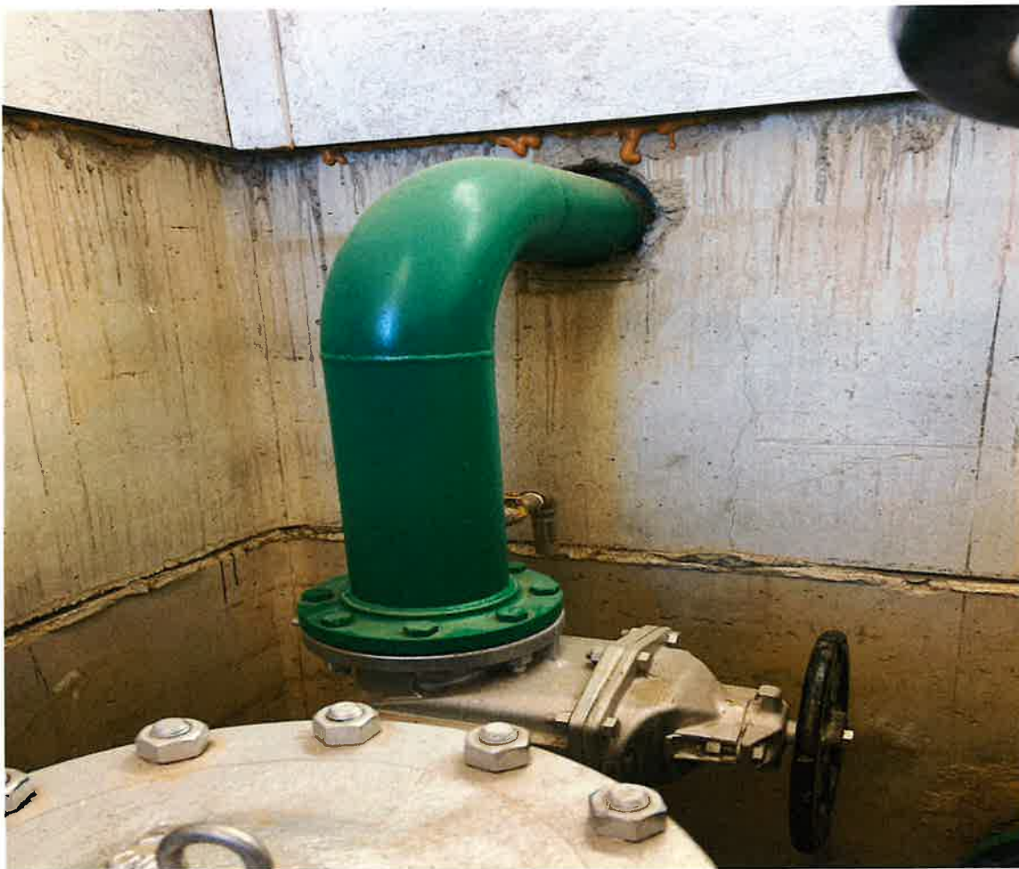
Fig. 14 – Close up of pipe coming from storage tanks to plant.
