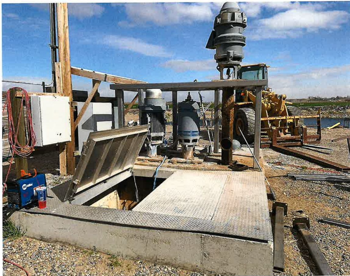
Fig. 22 – Three 100 hp pumps deliver the waste water to the pivots.
