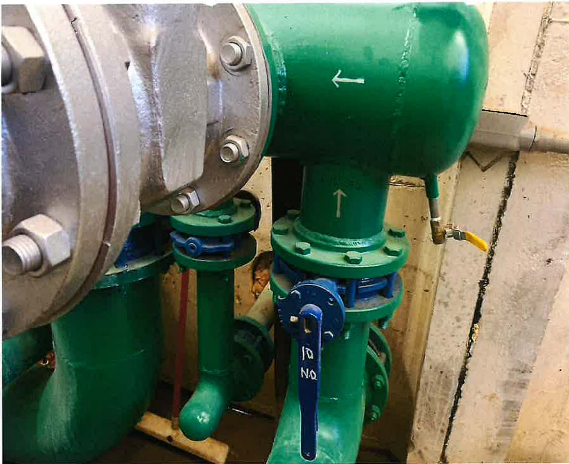
Fig. 11 - Each pipe is labeled with which well it is coming from when going to the storage tanks.
