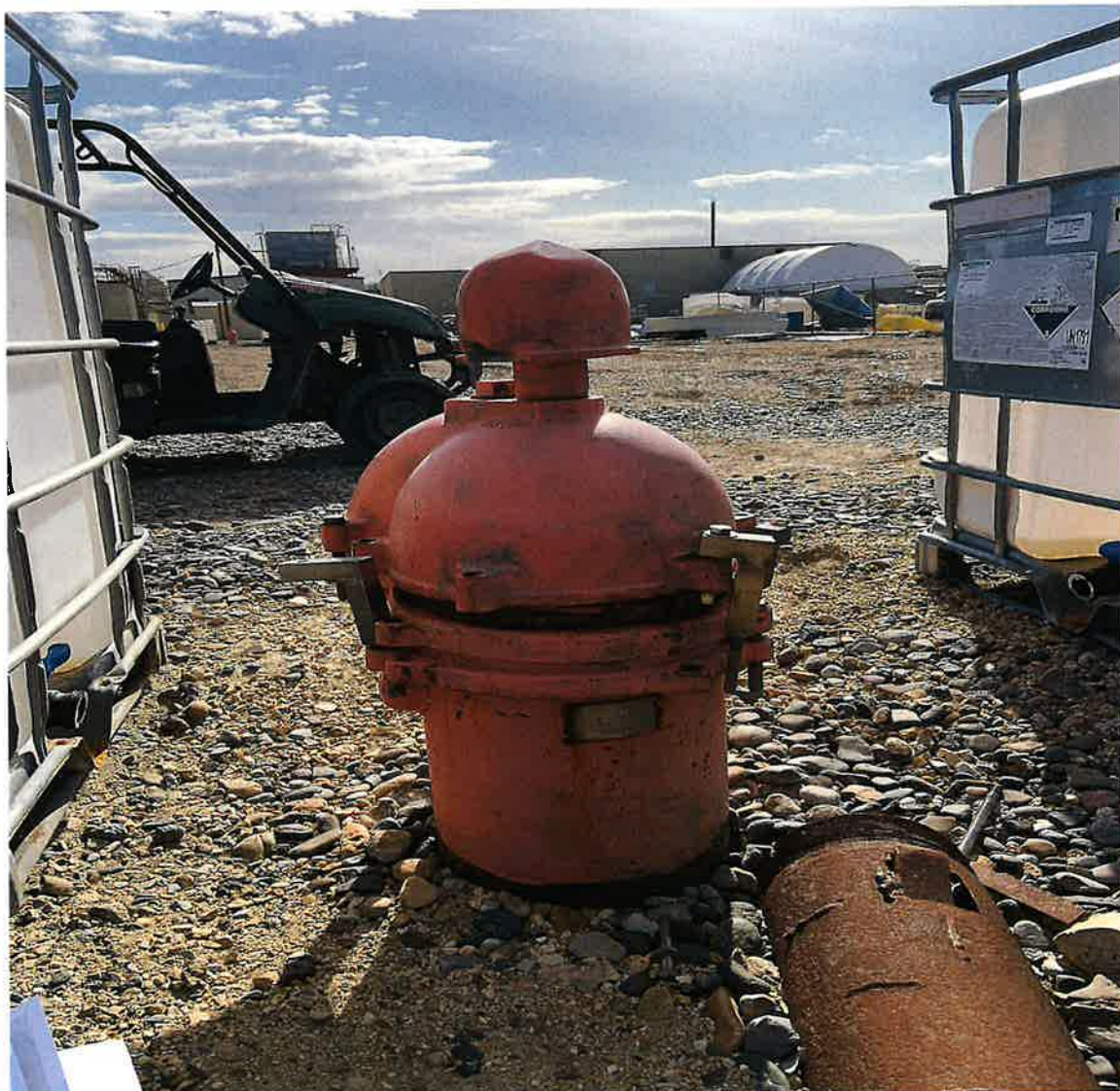
Fig. 4 - Well tag ID #D0031658 has a 10" casing from 3-400 ft bsl. All 5 wells feed water into the storage tanks which then deliver water to the plant.
