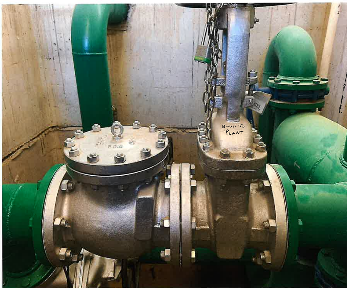
Fig. 12 – There is a bypass valve from the wells directly to the plant which is always closed and locked according to plant operators.
