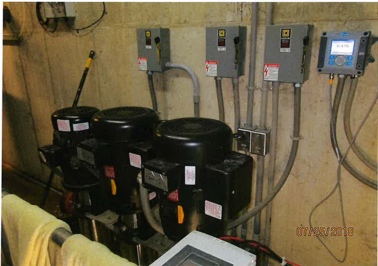
TWO 3HP PUMPS ASSOCIATED WITH DIVERSION SYSTEM
