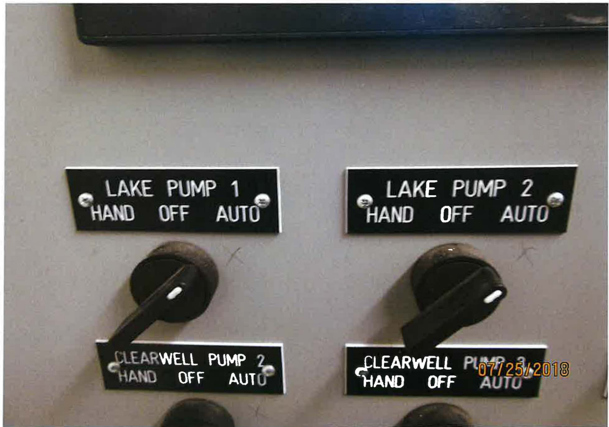
TWO 3 HP PUMPS – CONTROL PANEL
