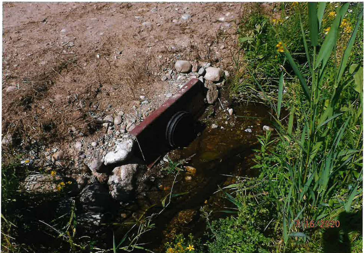
CAREYWOOD CREEK SIDE OF OVERFLOW DISCHARGE PIPE
