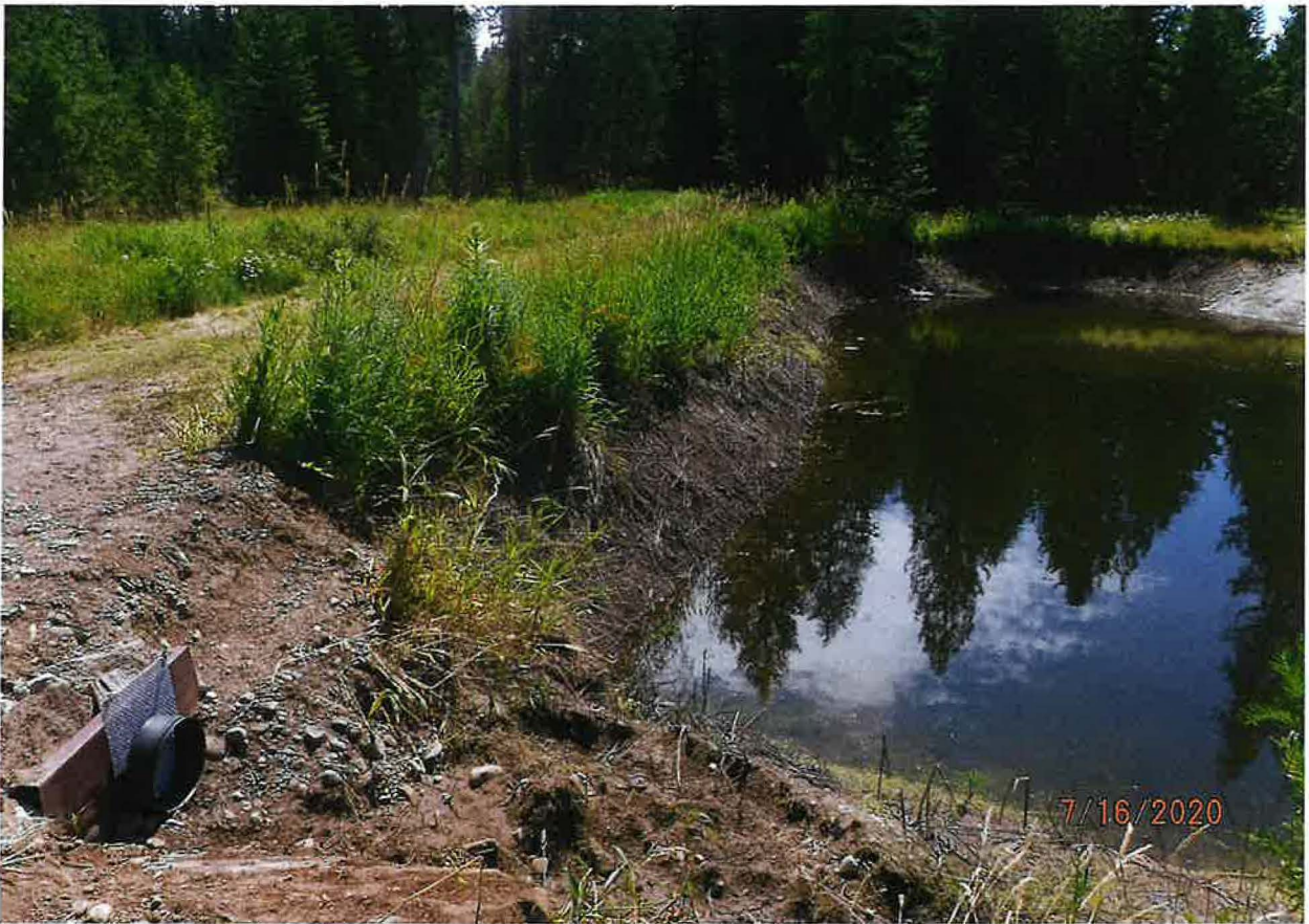
OVERFLOW DISCHARGE PIPE FROM POND TO CAREYWOOD CREEK
