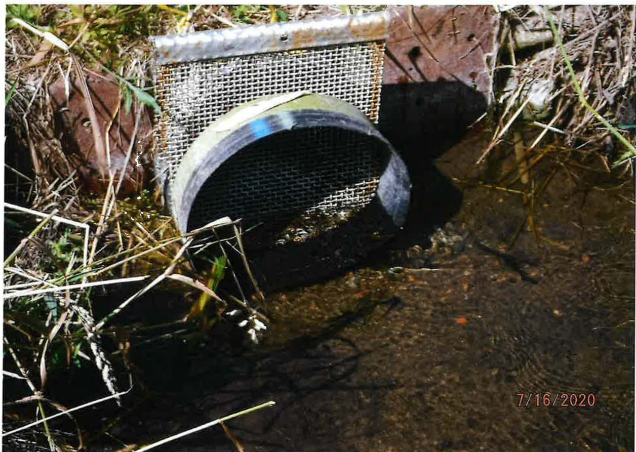
POD – 14 INCH CORRUGATED PIPE DIVERTING FROM CAREYWOOD CREEK
