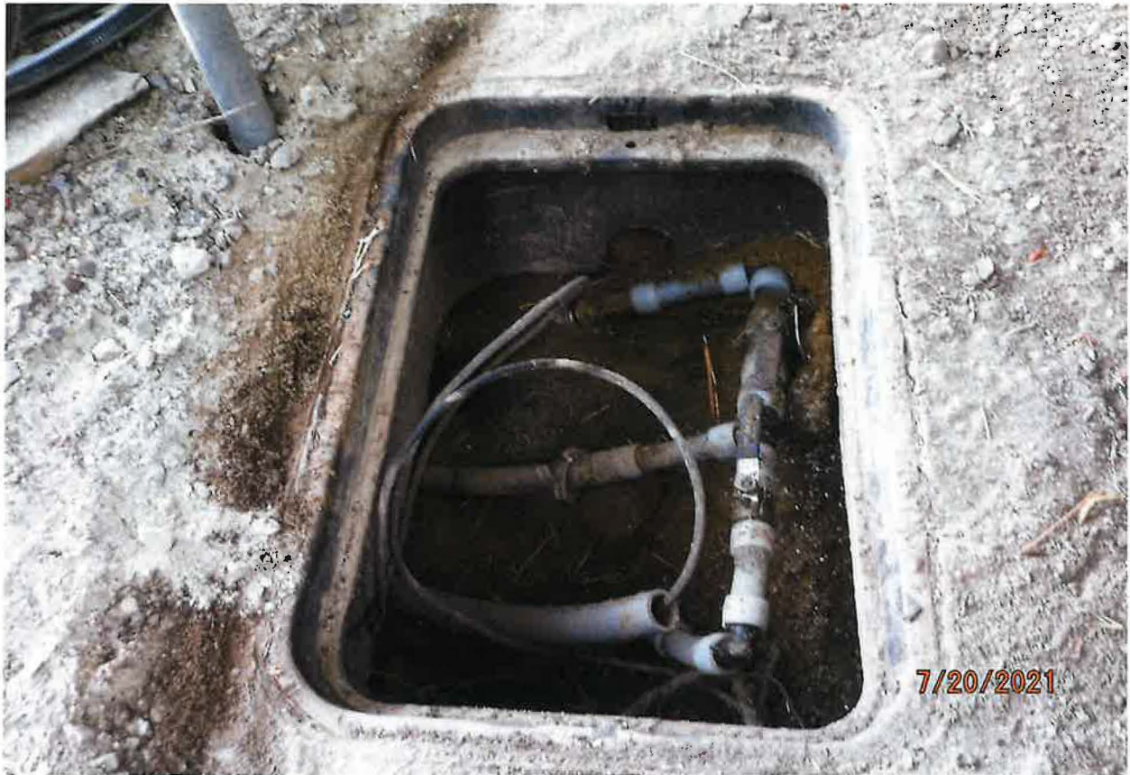
IRRIGATION SYSTEM CONTROL BOX – LOCATED NEXT TO FROST FREE HYDRANT
