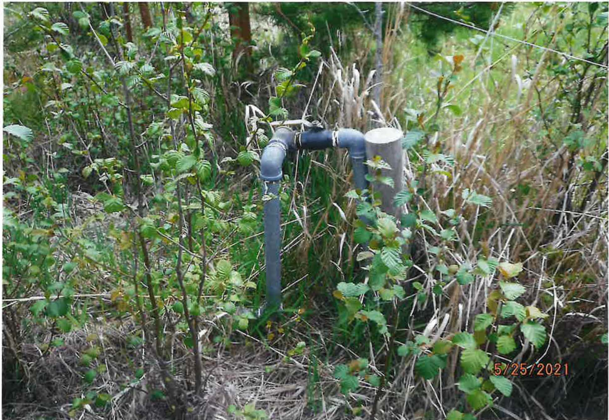
IRRIGATION POU – EAST SIDE OF CREEK – MAIN WATER LINE
