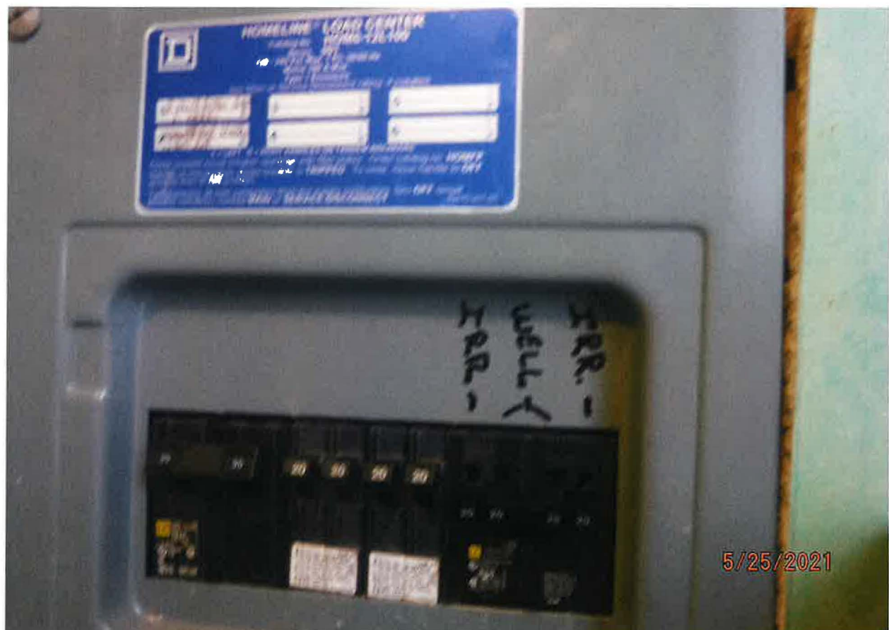
CIRCUIT BREAKERS USED TO CYCLE SYSTEM BETWEEN TWO WELL PUMPS
