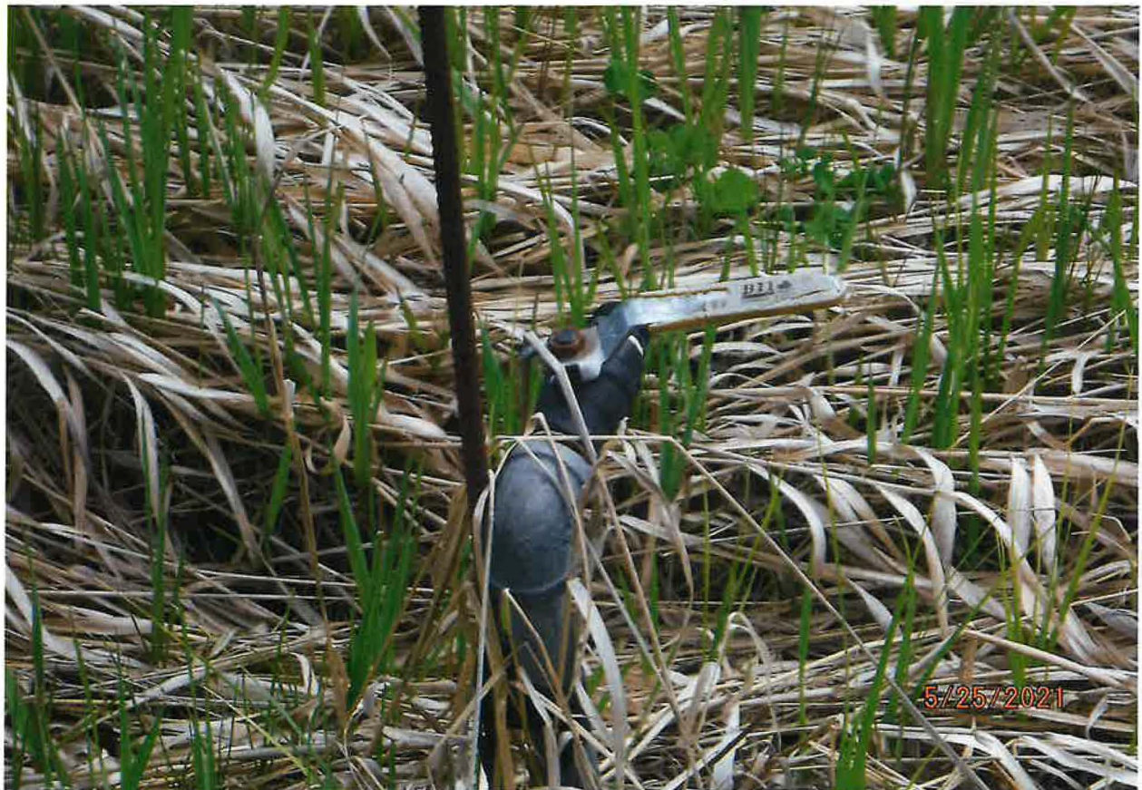
IRRIGATION RISERS OFF MAIN WATER DISTRIBUTION PIPE
