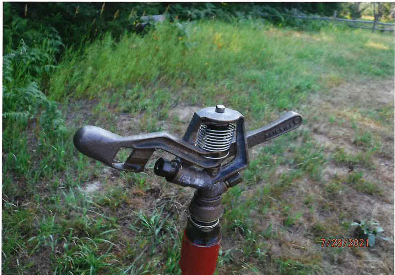
RAINBIRD TRIPOD SPRINKLERS WITH 11/64 NOZZLE USED AT IRRIGATION POU
