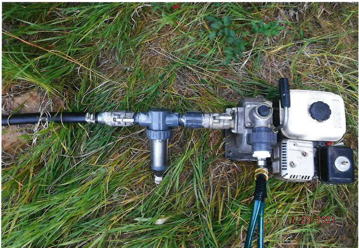
1.5 INCH POLY PIPE INTAKE LINE TO PUMP TO HOSE BIB SPLITTER
