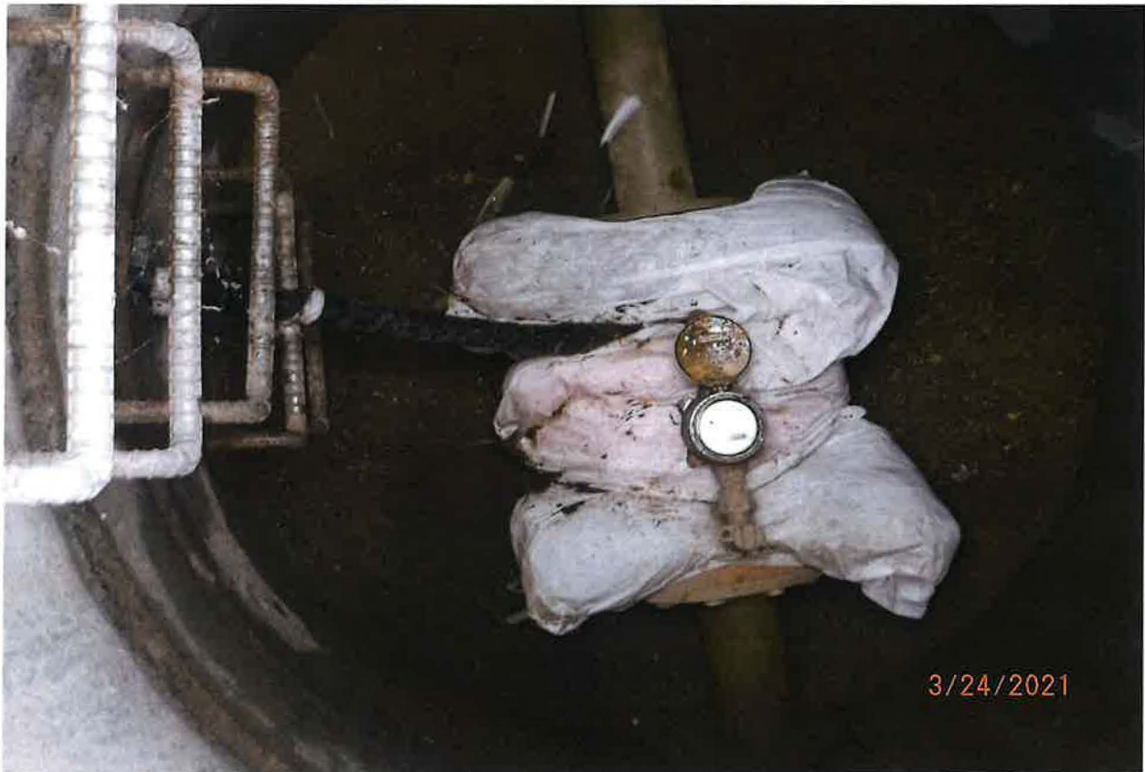
1 OF 2 EA MAIN LINE VALVES DISCONNECTED – TERMINATES WATER SERVICE TO NEWPORT, WA
