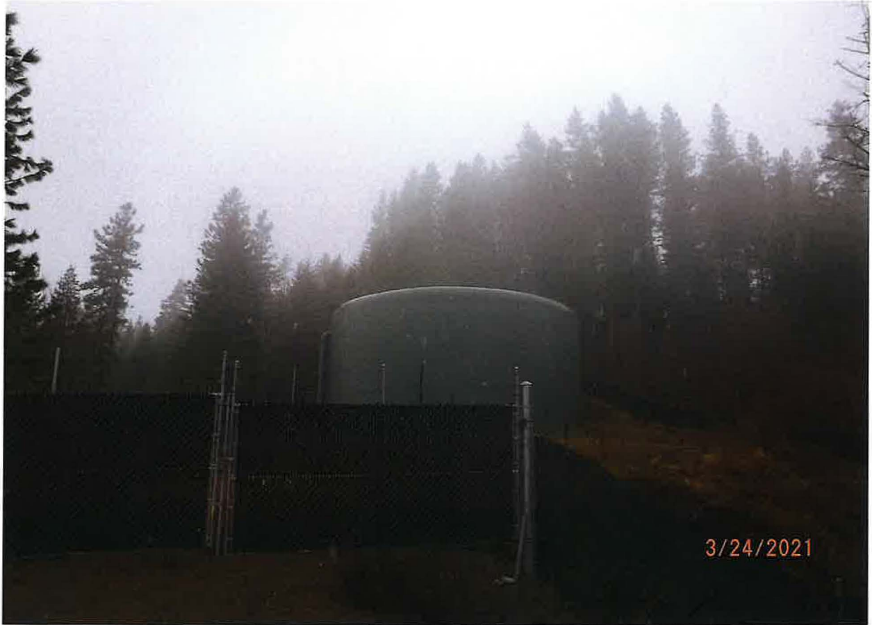
1 MILLION GALLON STORAGE TANK ASSOCIATED WITH 2 WELLS WATER CONVEYANCE SYSTEM
