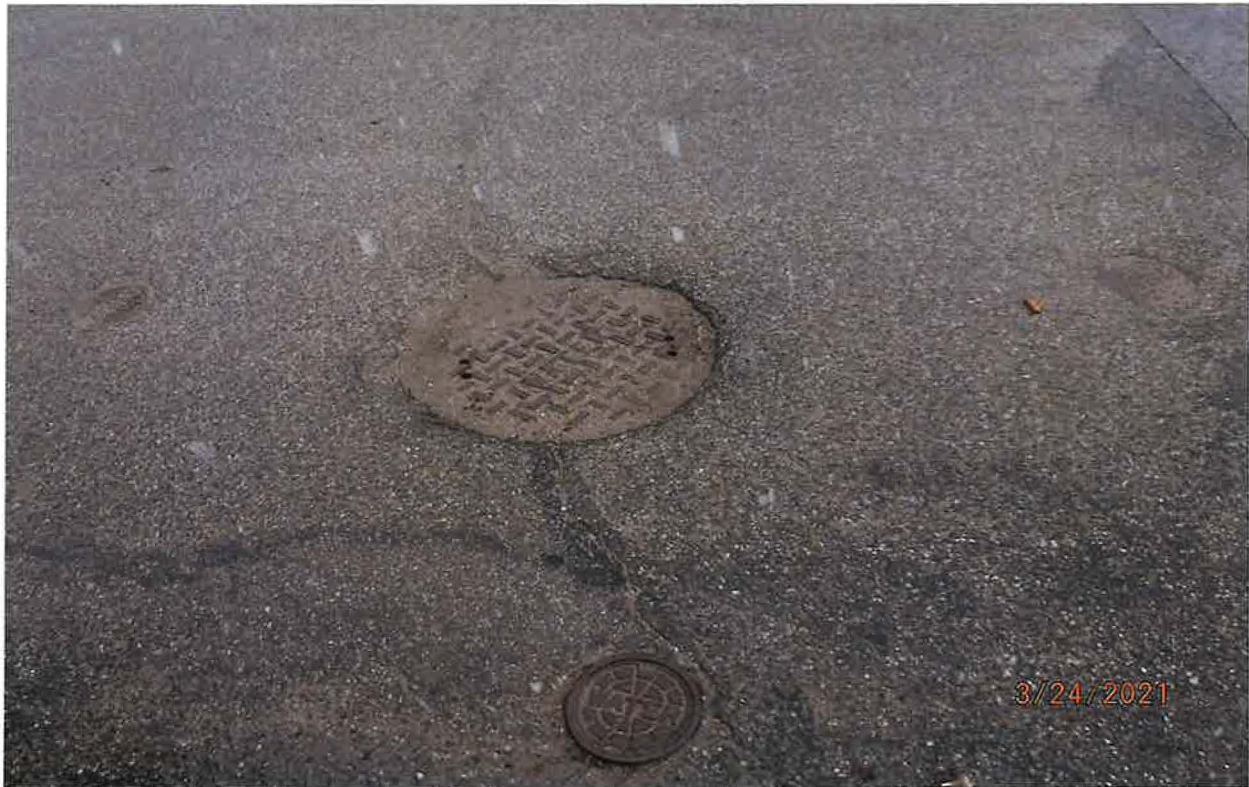
2 OF 2 EA MAIN LINE VALVES (LOCATION) DISCONNECTED – TERMINATES WATER SERVICE TO NEWPORT, WA
