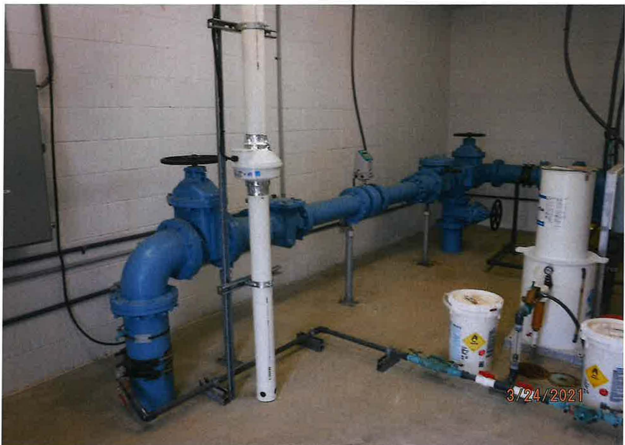
WATER CONVEYANCE SYSTEM – WATER MAIN FROM EAST WELL
