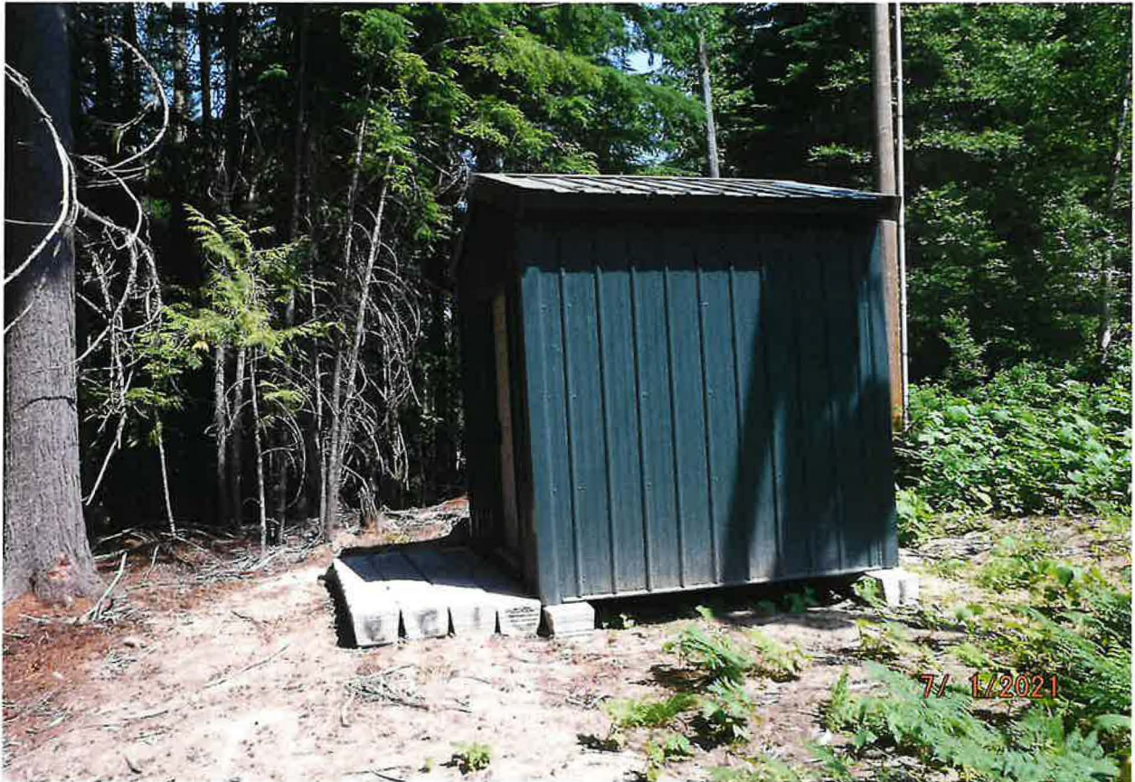
PUMP CONTROL HOUSE FOR WELL No.2
