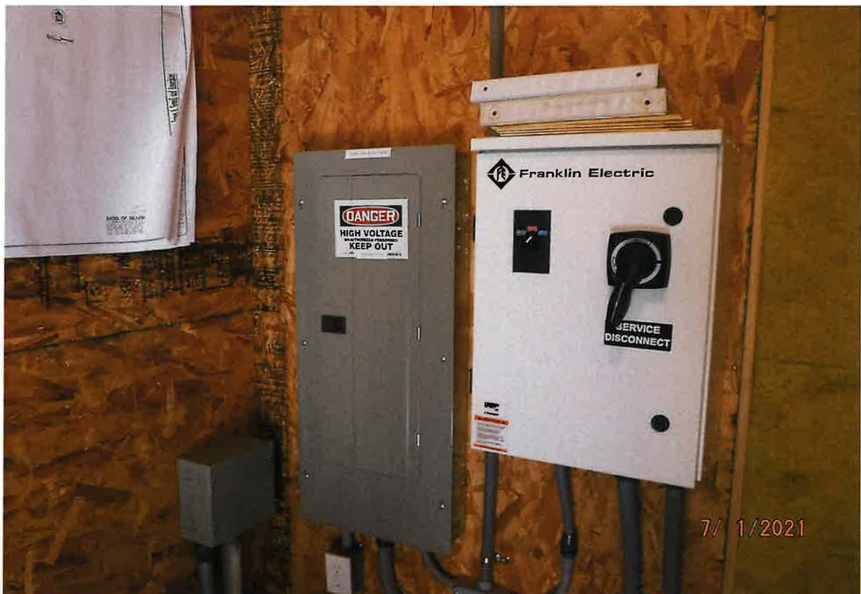
7/7.5 HP, 3 PHASE PUMP INSTALLED IN WELL No.2 D0028727
