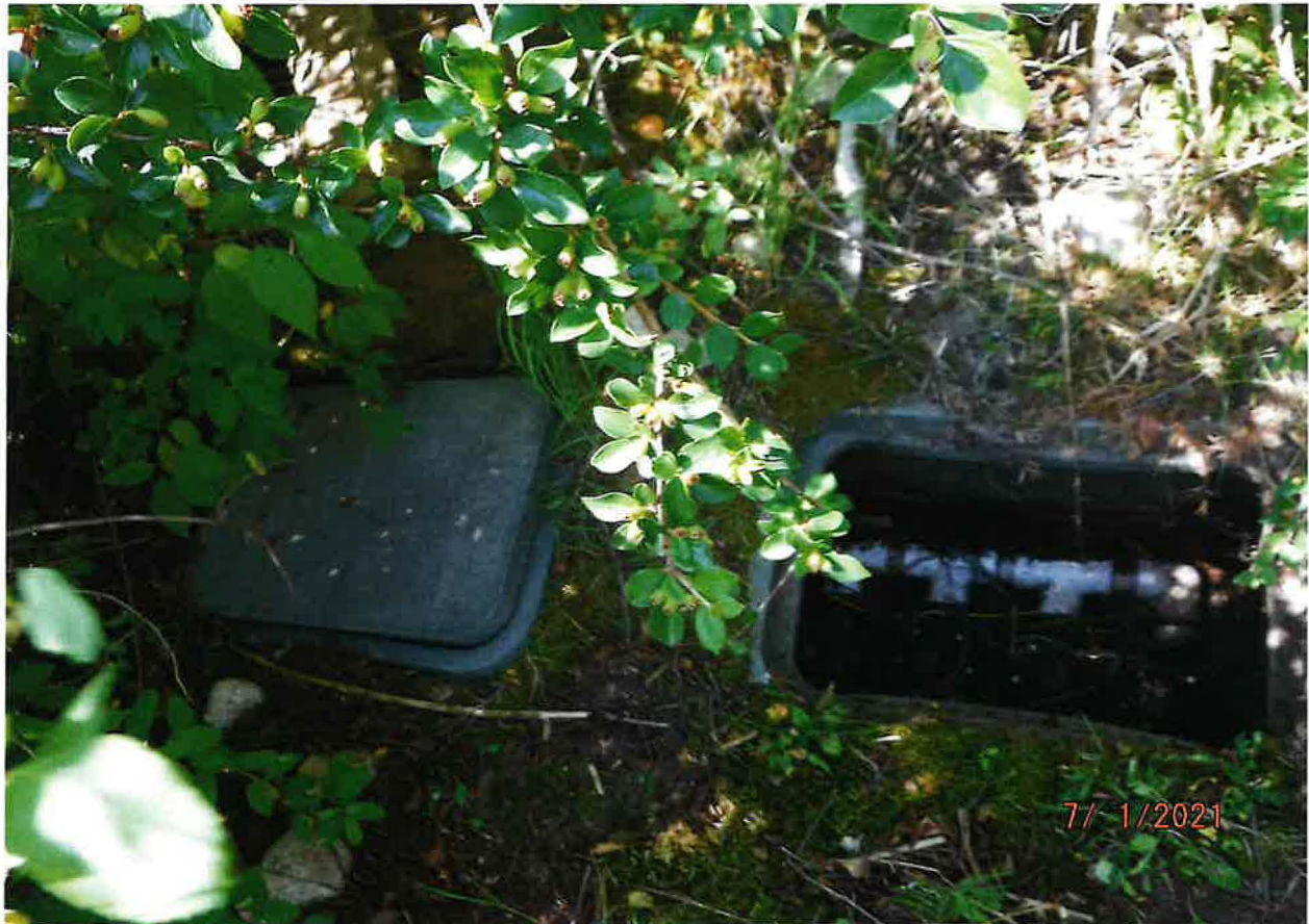
8 STATION PRESSURIZED SPRINKLER CONTROLS LOCATED SOUTH OF HANGER
