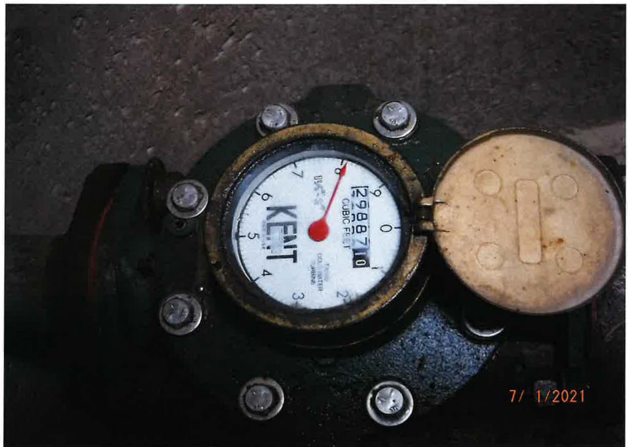
KENT FLOWMETER INSTALLED ON MAIN LINE FROM WELL No.1
