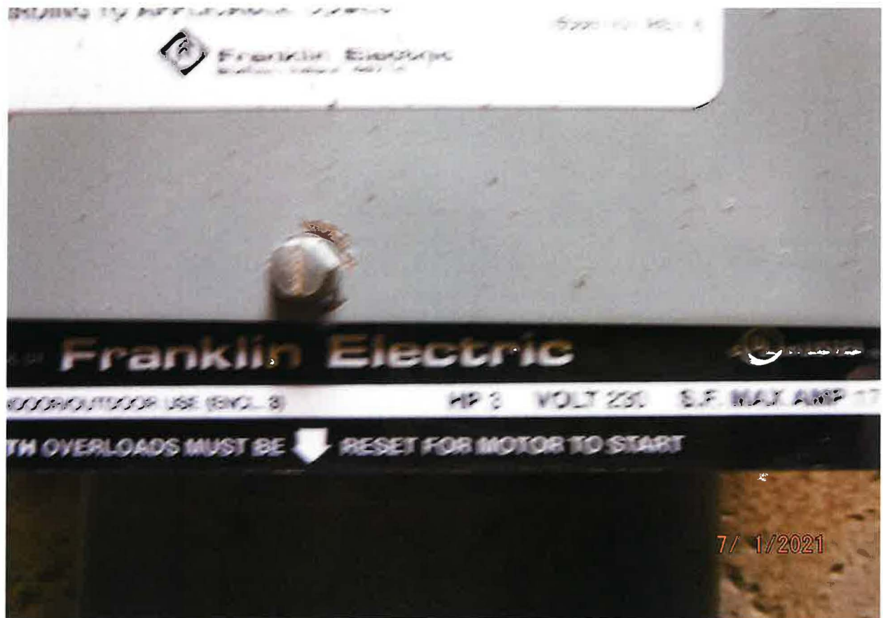
3 HP PUMP INSTALLED IN WELL 97-93-N-31-000
