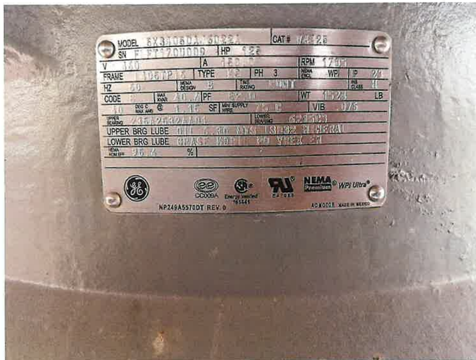
Pump Motor Name Plate
