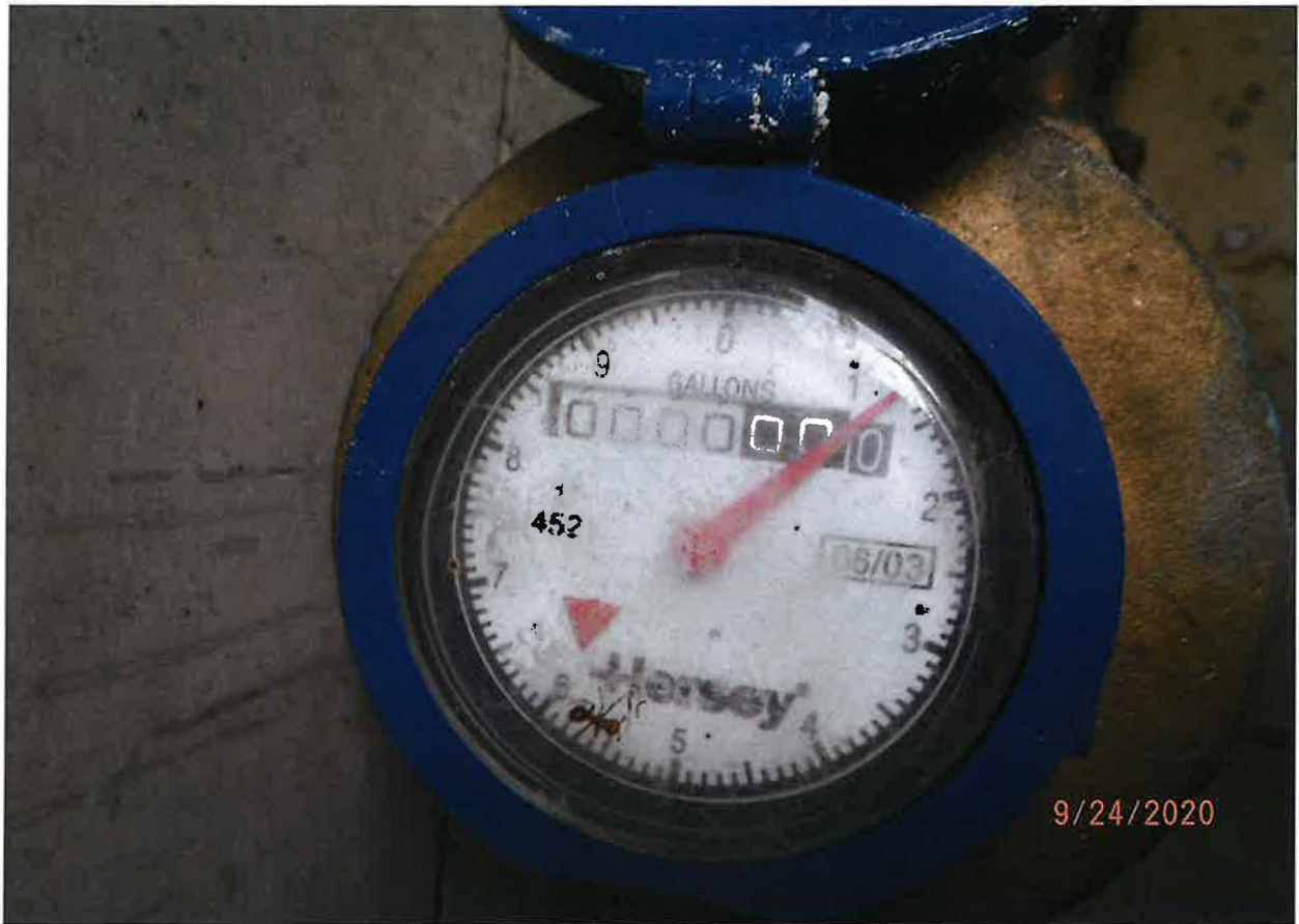
2EA FLOW METERS INSTALLED TO CAPTURE VOLUME READINGS IN PUMP CONTROL VAULT
