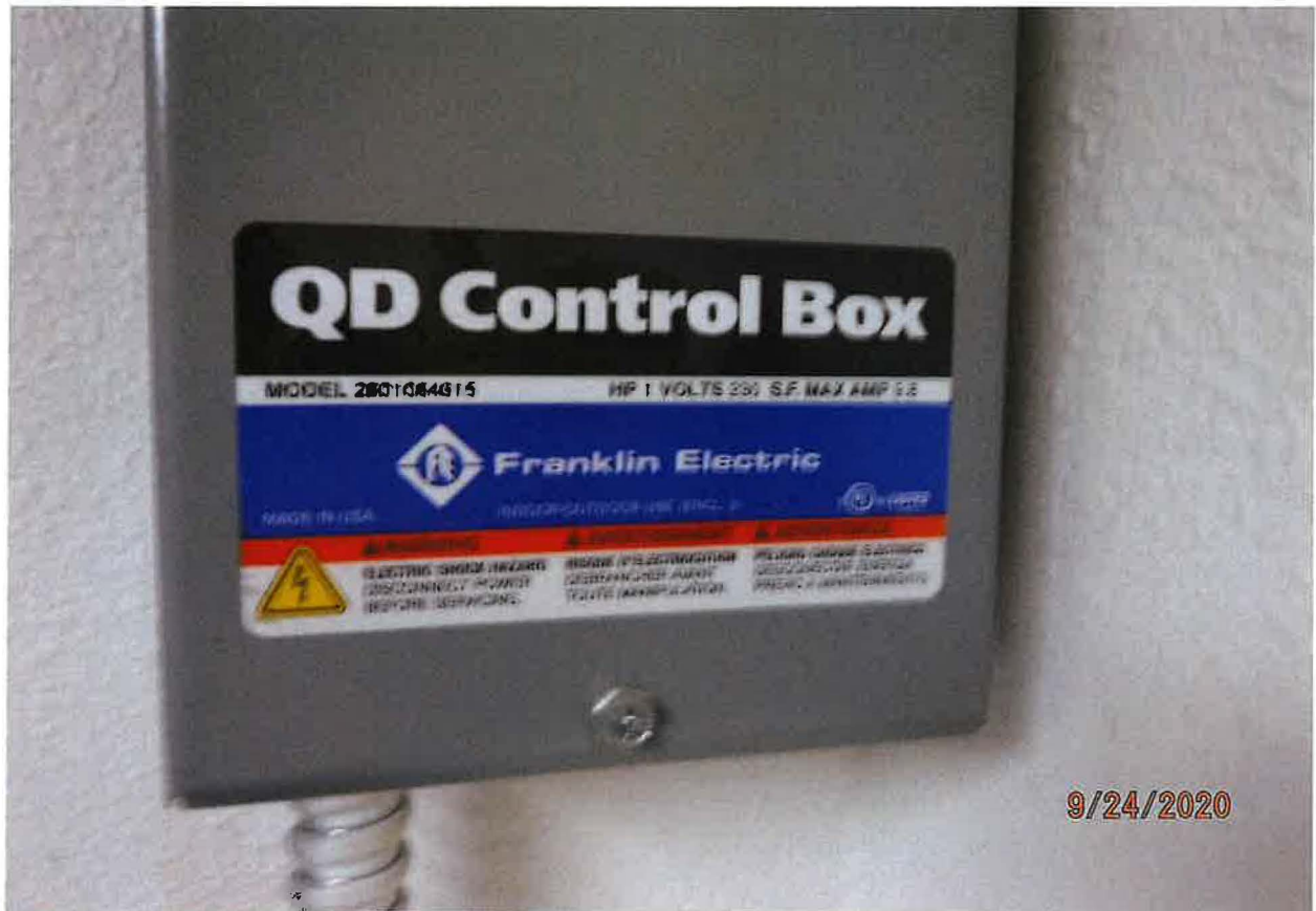
1 HP PUMP IN WELL 96-91-N-61
