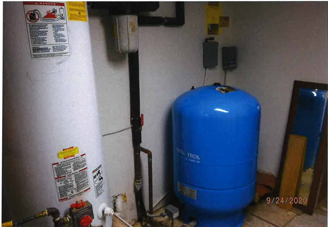
CARETAKER HOUSE PRESSURE TANK AND PUMP CONTROLLER
