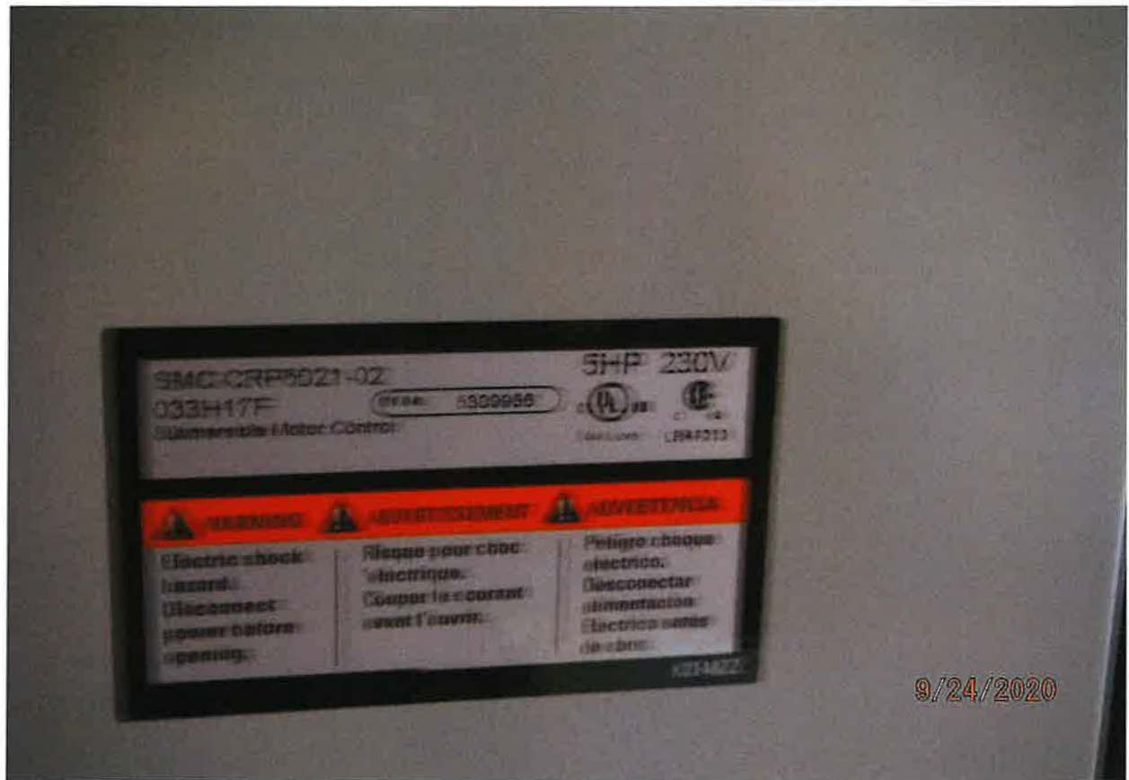
5 HP PUMP IN WELL WITHOUT TAG
