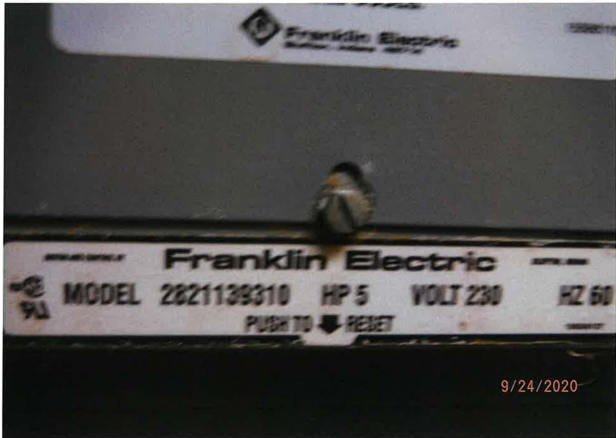
5 HP PUMP IN WELL D0054541
