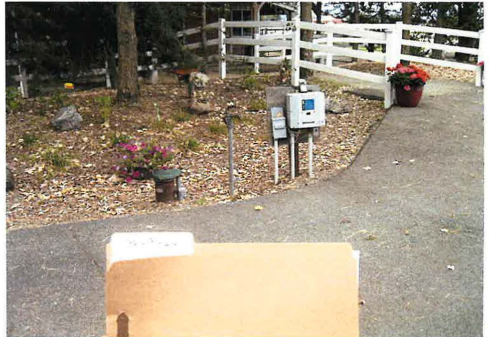
Well DØØ41314 & zone control box
