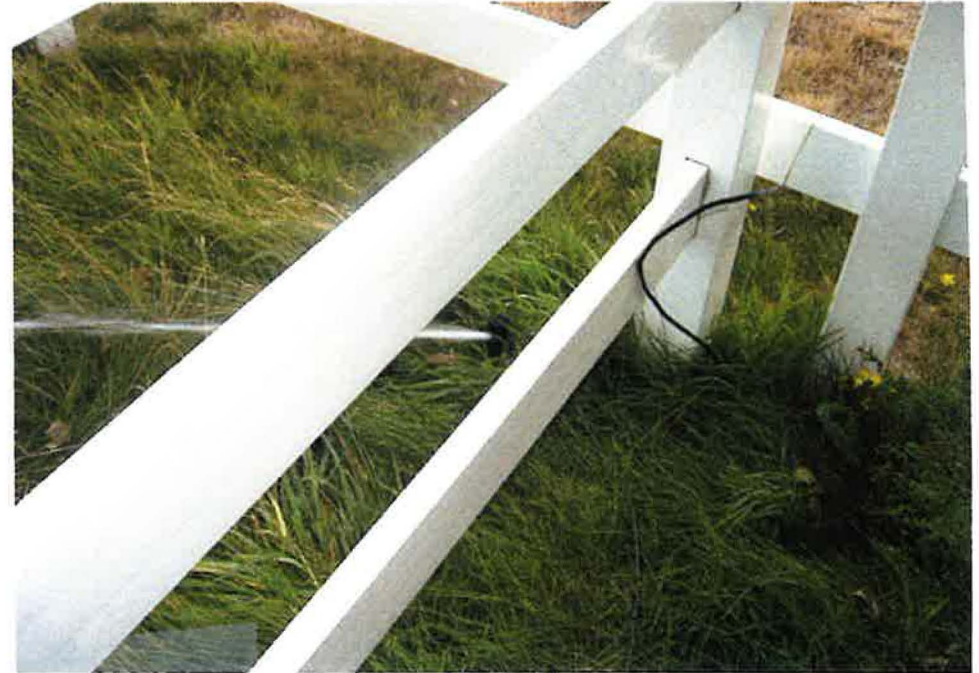
Fence corner with operating sprinkler.
