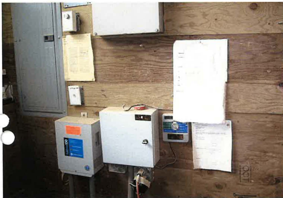
Irrigation timer & zone controls in Indoor Arena.
