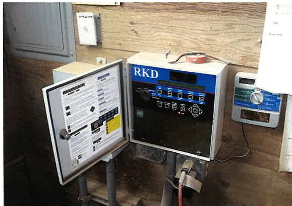
Opened Irrigation Zone control box. (No real time flow rate)
